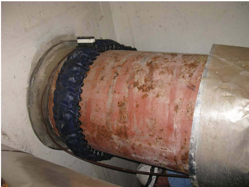
Figure 3.7: Location 2, Service Water Valve Pit
