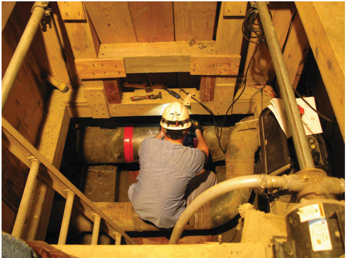
Figure 3.16: Location 5, 12-inch Line in an excavation in the AFP Building
