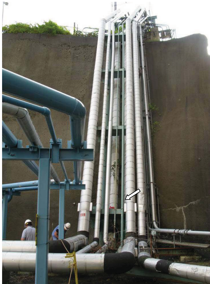
Figure 3.19: Location 6, 12-inch Line from CST to AFP Building
