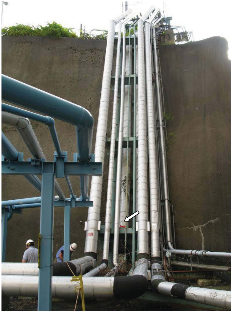
Figure 3.10: Location 3, 8-inch Line from the AFW Building up to CST
