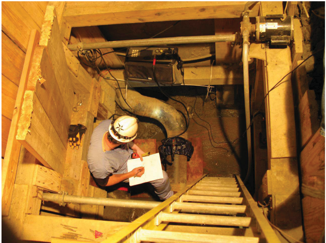
Figure 3.13: Location 4, 8-inch Line in an excavation in the FRV Building
