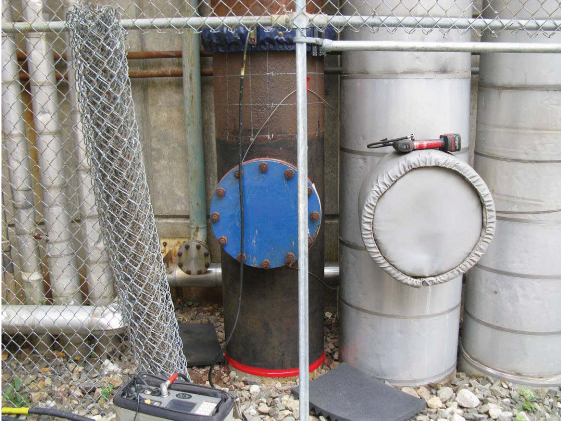
Figure 3.1: Location 1, Service Water Header, Transformer Yard
