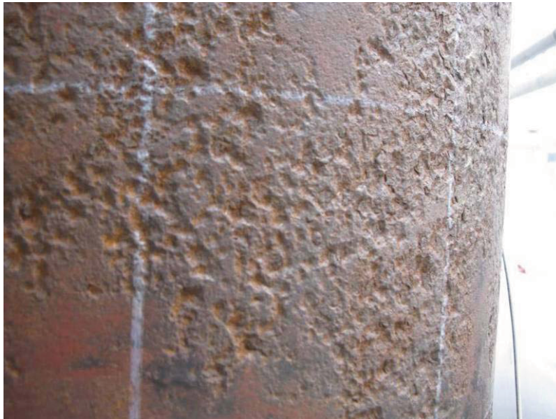
Figure 3.2: Location 1, Service Water Header, Under Insulation Corrosion
