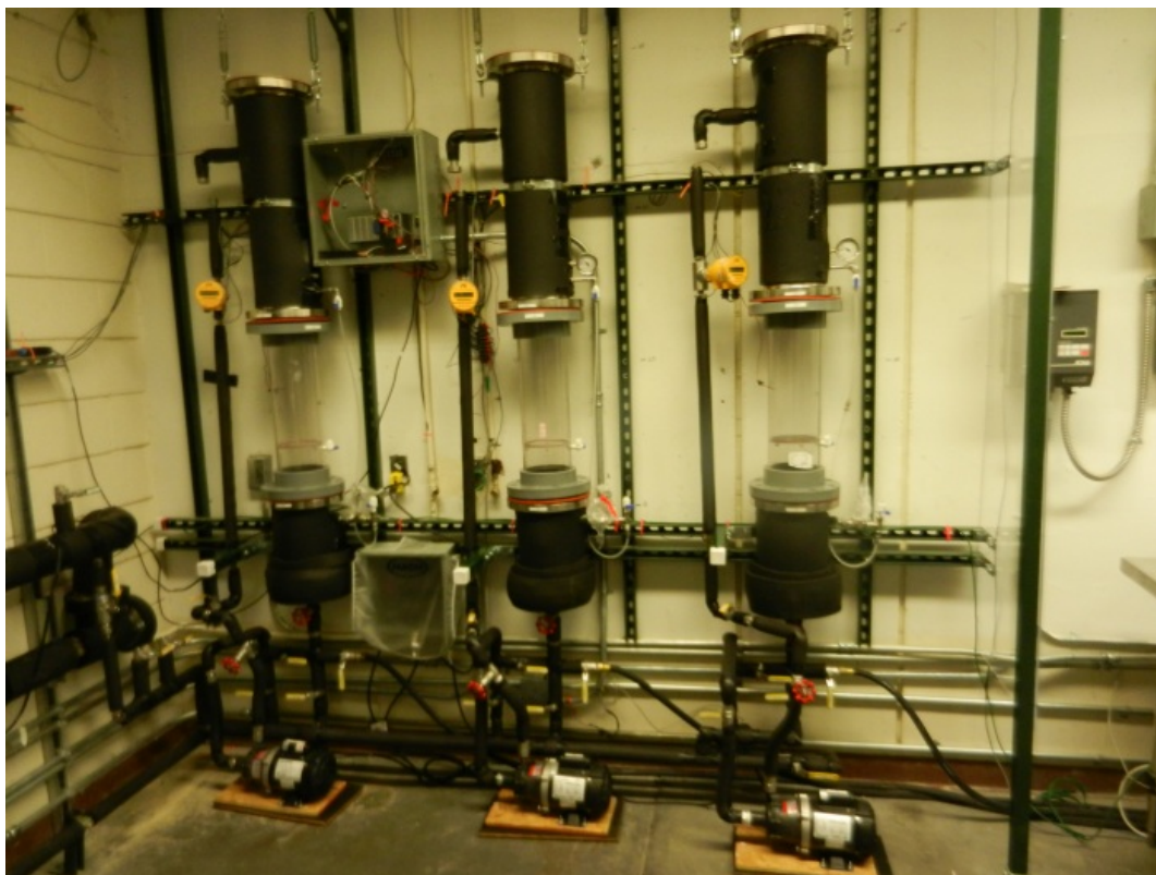
Figure 4 – CHLE Head Loss Columns.
