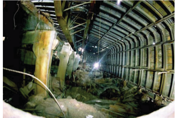
FIG. 7.3. Reactor room of unit 4 after the accident.
