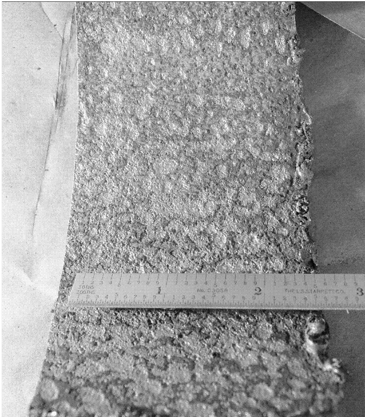
Figure 36 – Inside surface of the pipe after cleaning showing superficial general corrosion.
