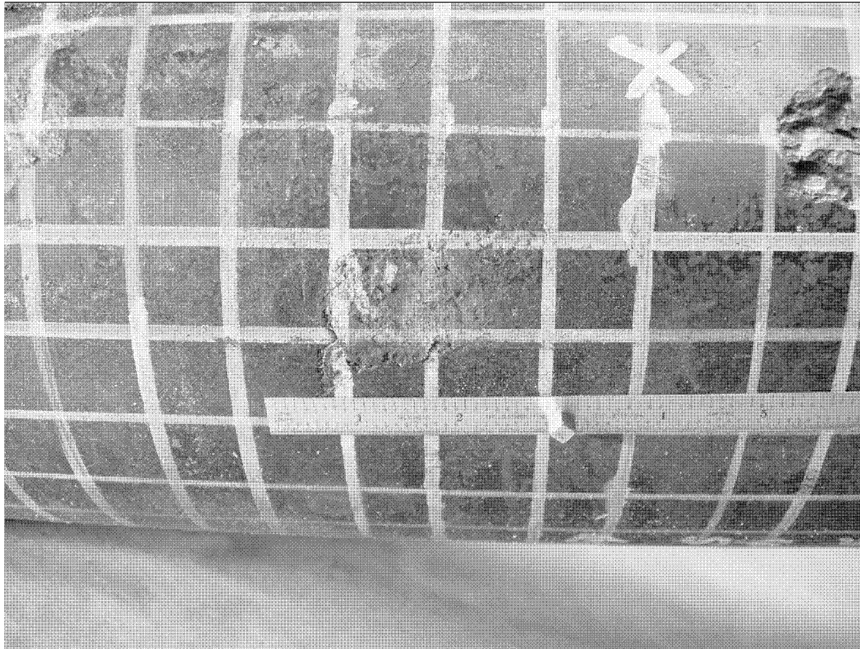
Figure 27 – External corrosion pit in the pipe (as-received condition) designated Area 11. Note absence of corrosion around the pit. In this example the corrosion product fills the area of metal loss so that the corrosion product surface is nearly flush with the pipe surface. See next figure for detail
