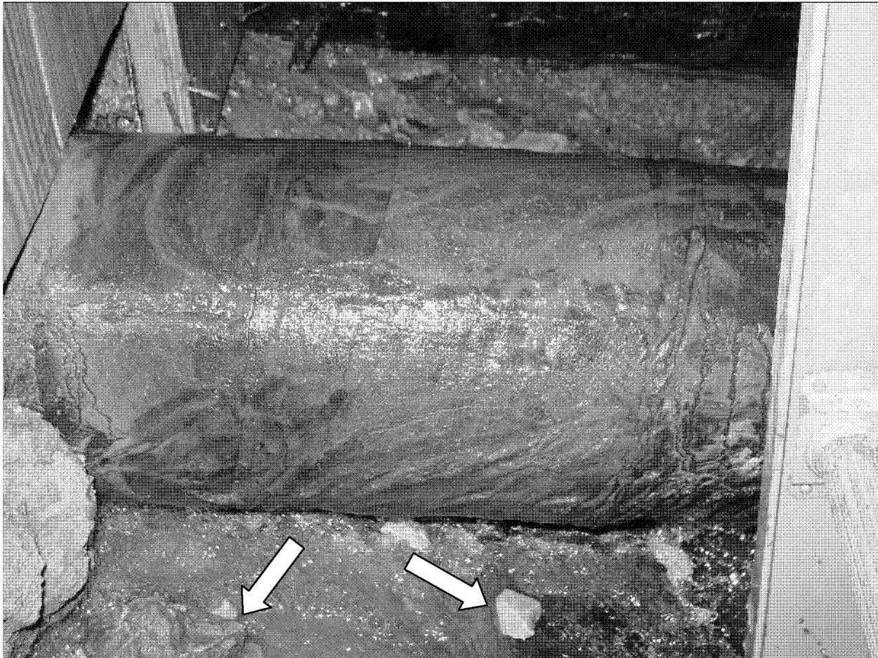
Figure 1- View of pipe coating as observed in the excavation by Entergy Staff
