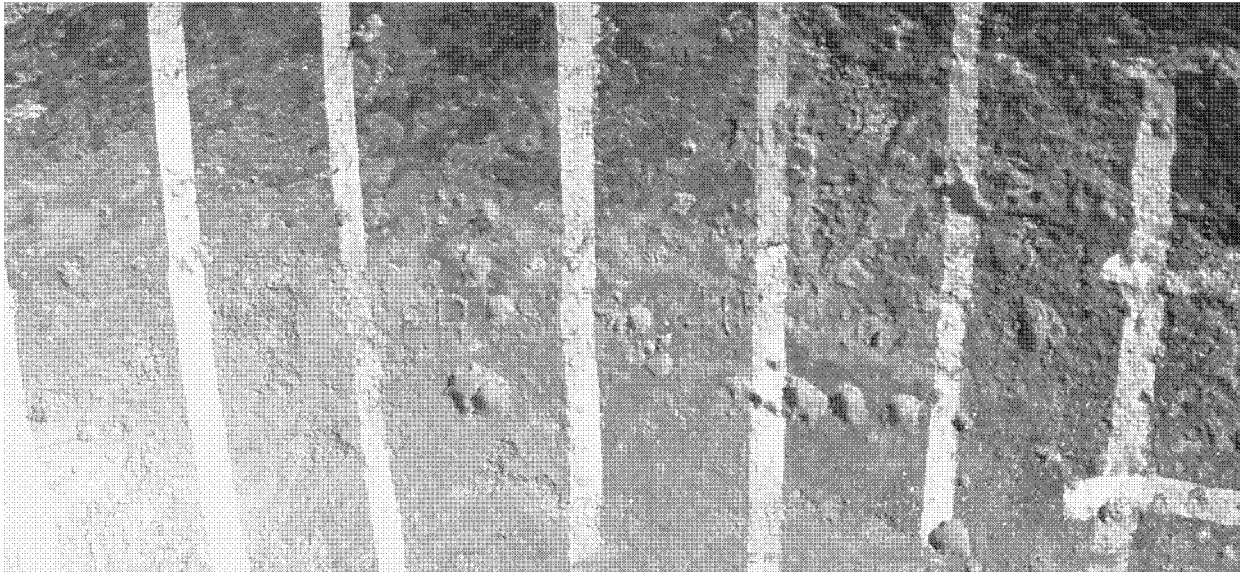
Figure 13 - Manufacturer's stamp marks on the neutral axis of the elbow. See next figure for detail of the stamp mark after cleaning.
