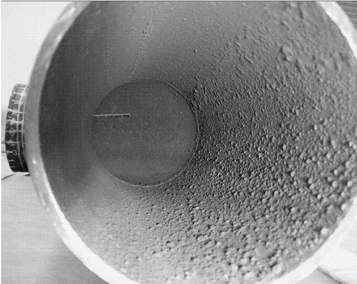
Figure 33 – Inside view of pipe sample looking from straight pipe toward the elbow (as received condition).
