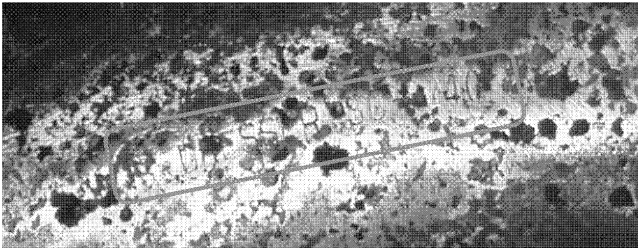
Figure 14 - Manufacturer's stamp mark after light abrasion with sandpaper. The stamp marks on the neutral axis of the elbow identify it as an 8" schedule 40 fitting manufactured by Dresser. The grade of the fitting is obscured by corrosion.
