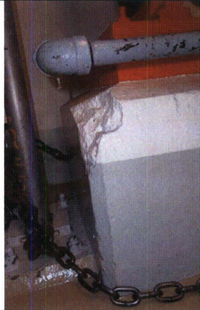
Note: Chipped concrete on corner of pump pedestal.
