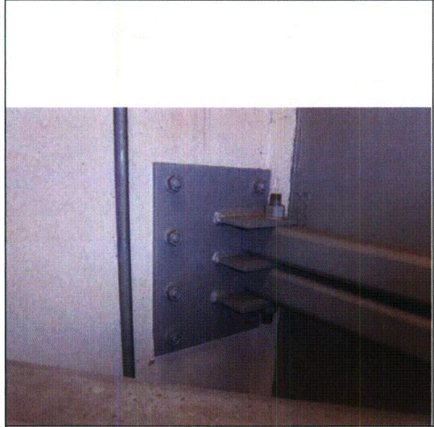
Note: Equipment anchorage for seismic restraining brace.
