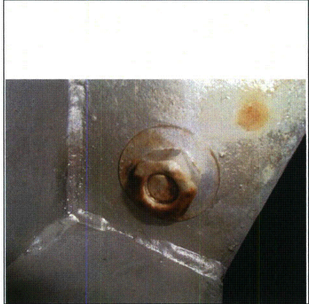
Note: Rusted bolt lacking full thread engagement (bottom view).
