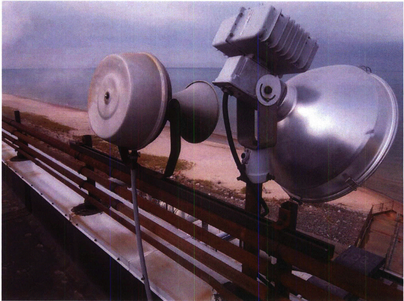
Sound and Lighting Located Above T-2, Taken From the Turbine Building.
