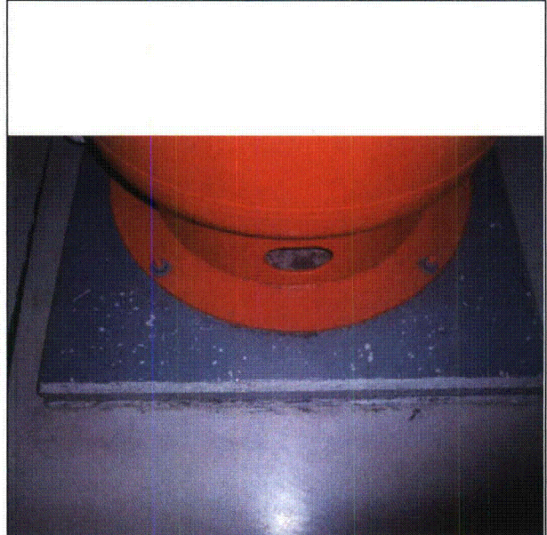
Note: Equipment anchorage.
