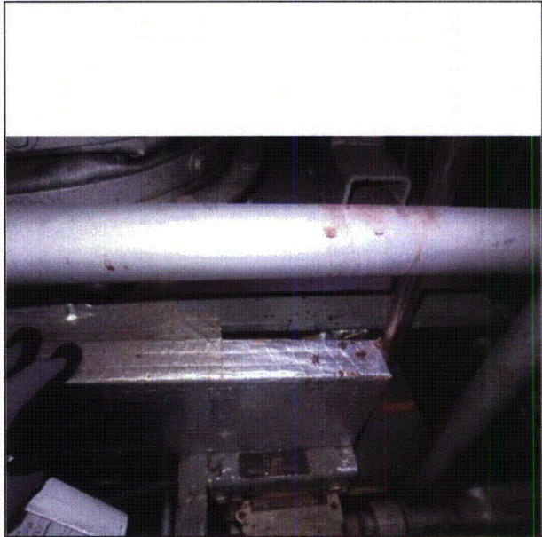
Note: Insulation separated from damper unit.
