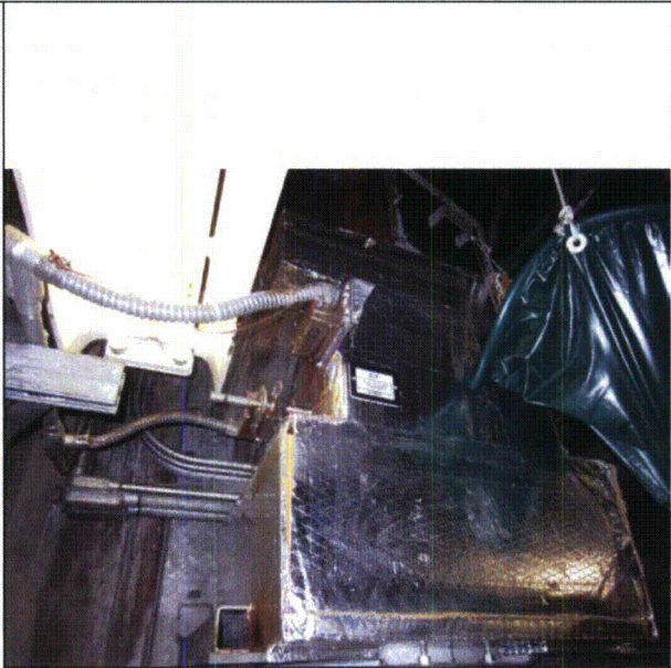
Note: Drip funnel overhead.
