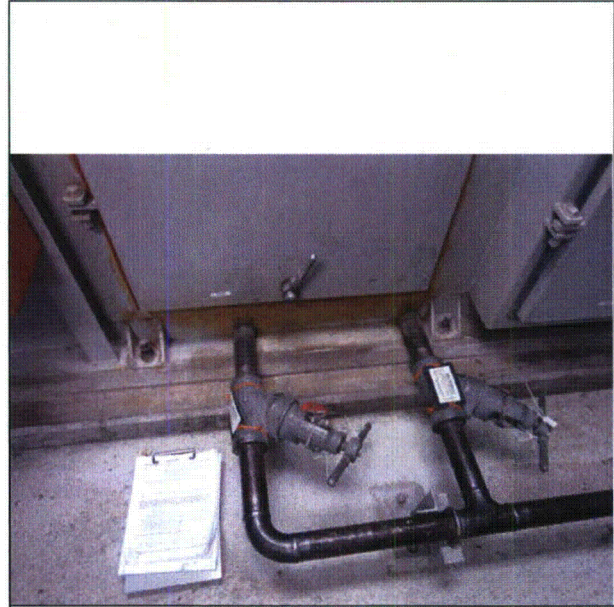
Note: Equipment Anchorage.
