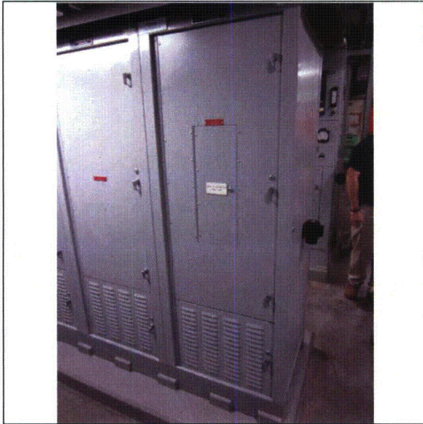
Note: Back panel of equipment.
