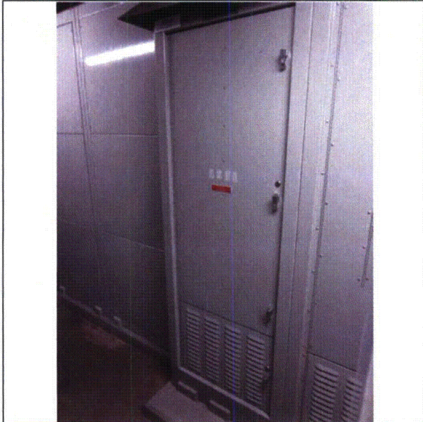
Note: Back panel of equipment.
