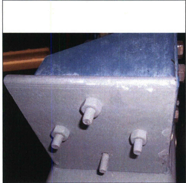
Note: Missing Nut from Anchorage to Steel Shelf Angle
