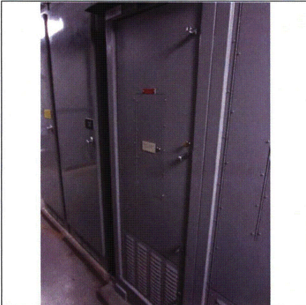
Note: Back panel of equipment.
