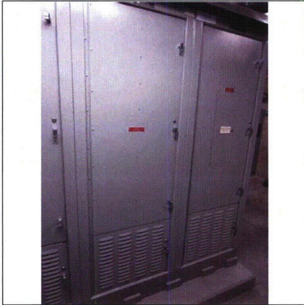
Note: Back panel of equipment.
