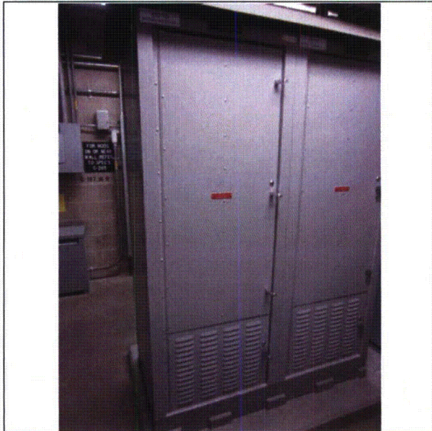
Note: Back panel of equipment.
