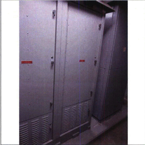
Note: Back panel of equipment.
