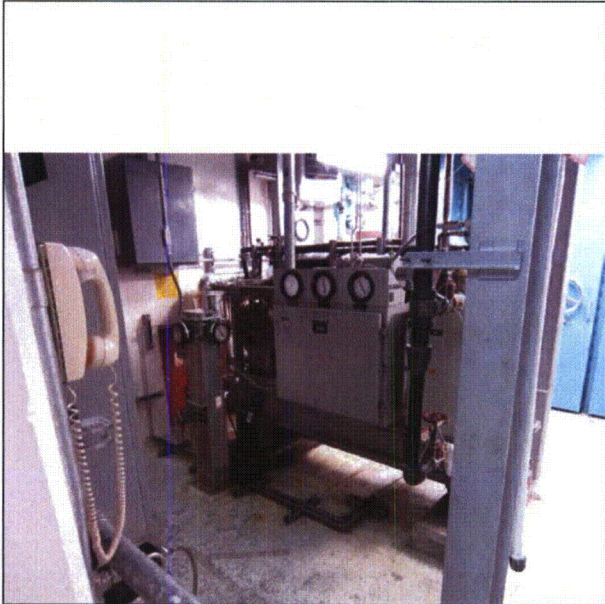
Note: Equipment view looking northwest.
