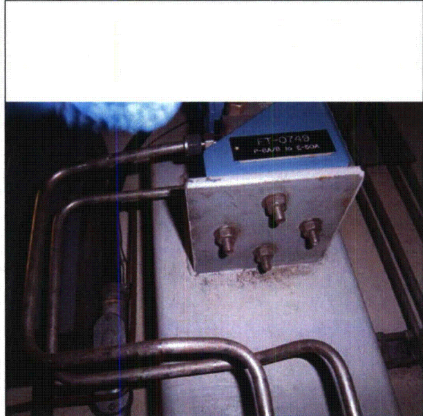
Note: Anchorage of equipment to shelf angle.
