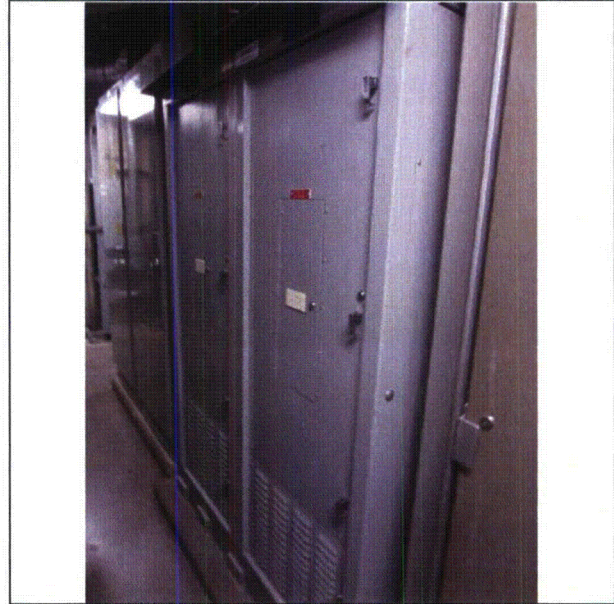
Note: Back panel of equipment.
