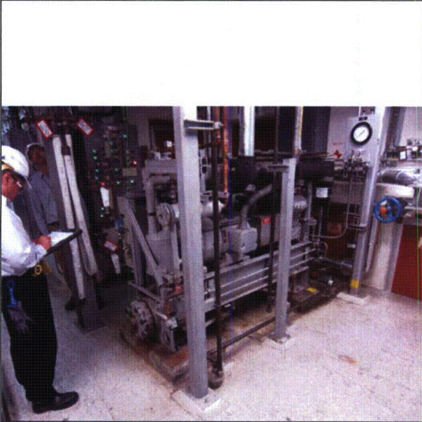
Note: Equipment view looking southwest.
