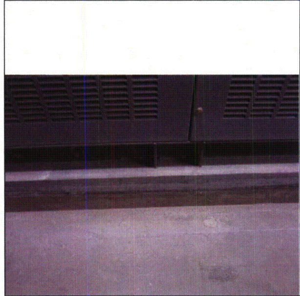
Note: Anchorage of equipment.
