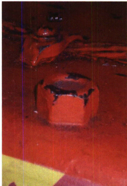
Note: Lack of Thread Engagement (West Center Bolt)
