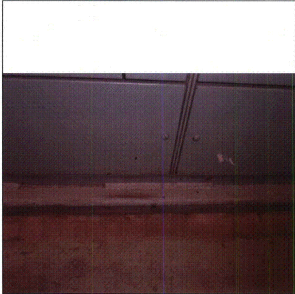
Note: Exterior Welds on Cabinet
