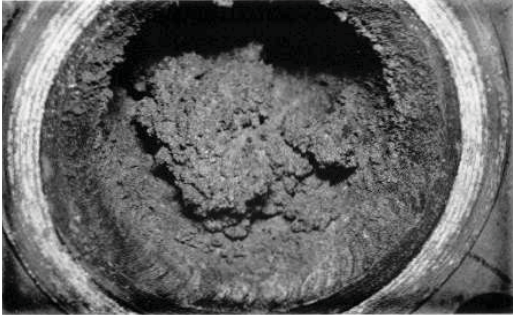
Figure D-7 Test LA3C, downstream end of pipe section 5 showing large bend deposit
