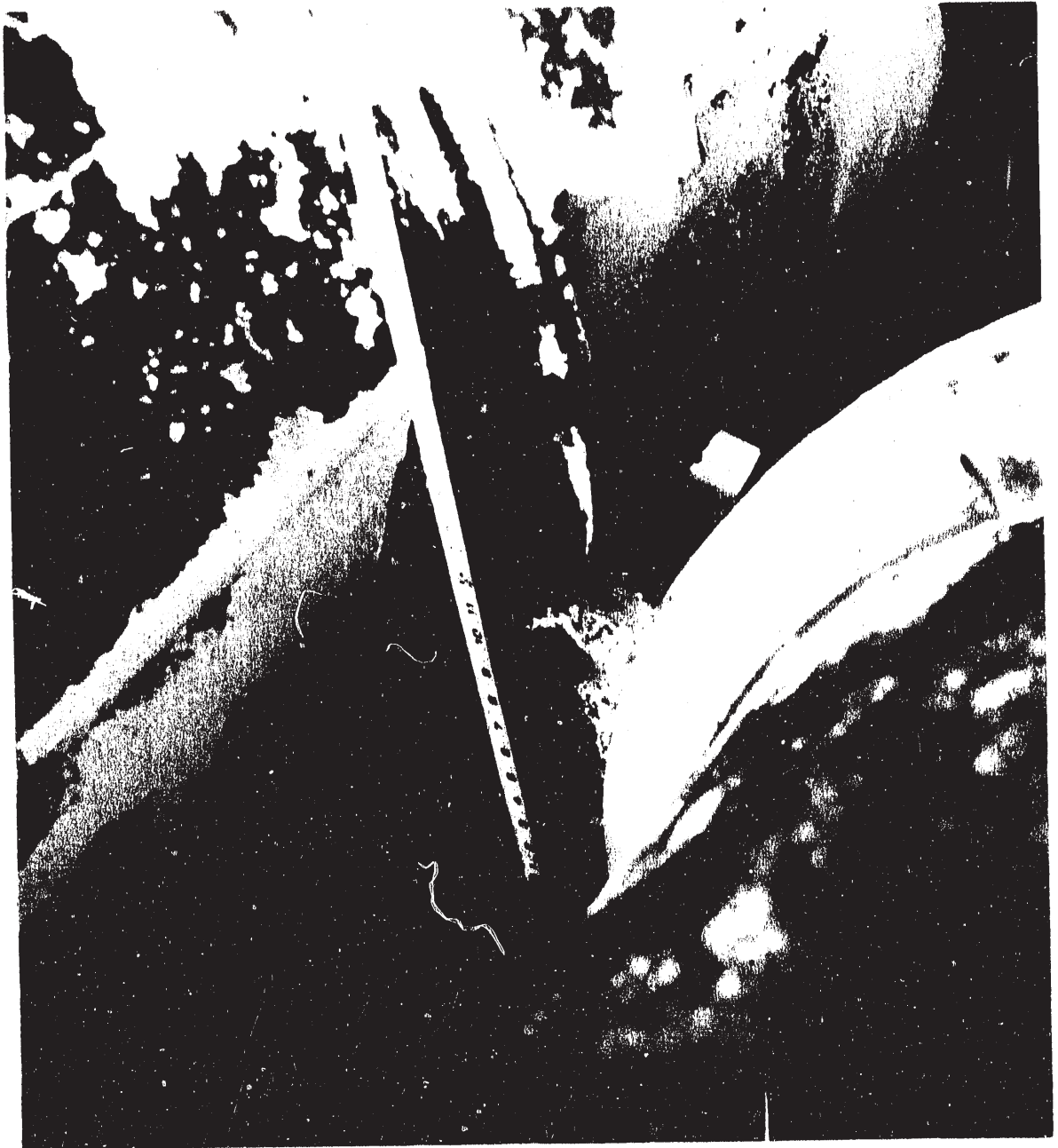
Fig. 3. Area of failure in cylinder 4G115688 showing relative position of lifting lug of neighboring cylinder.
