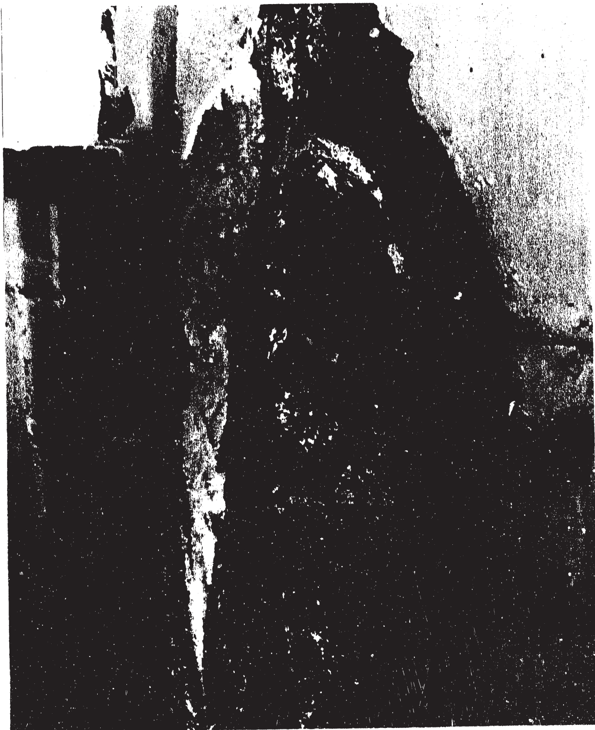
Fig. 4. Appearance of failure area on cylinder 4G127985 (after removal of debris covering hole).
