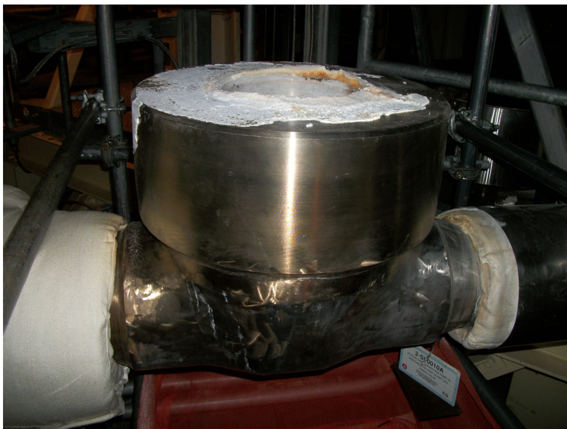
Figure 2: Photo of the enclosure
