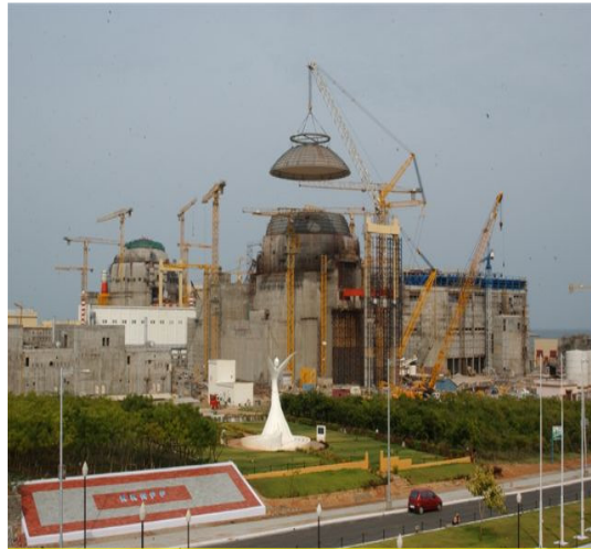
FIG. IV-4. Lifting the WWER-1000 containment dome into position at Kudankulam, India (Photo credit: NPCIL).
