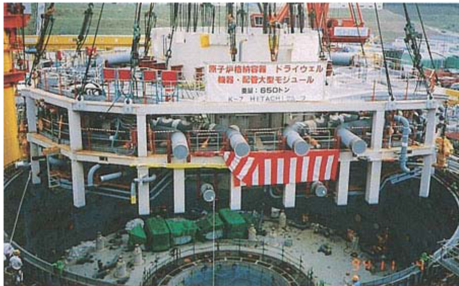
FIG. IV-7. Installing the upper drywell super large scale module at Kashiwazaki Kariwa-7 in Japan.
