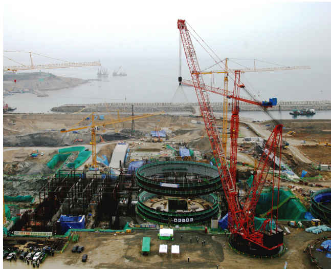
FIG. IV-9. Modularization of the containment liner plate assembly at Shin-Kori-1 in the Republic of Korea.
