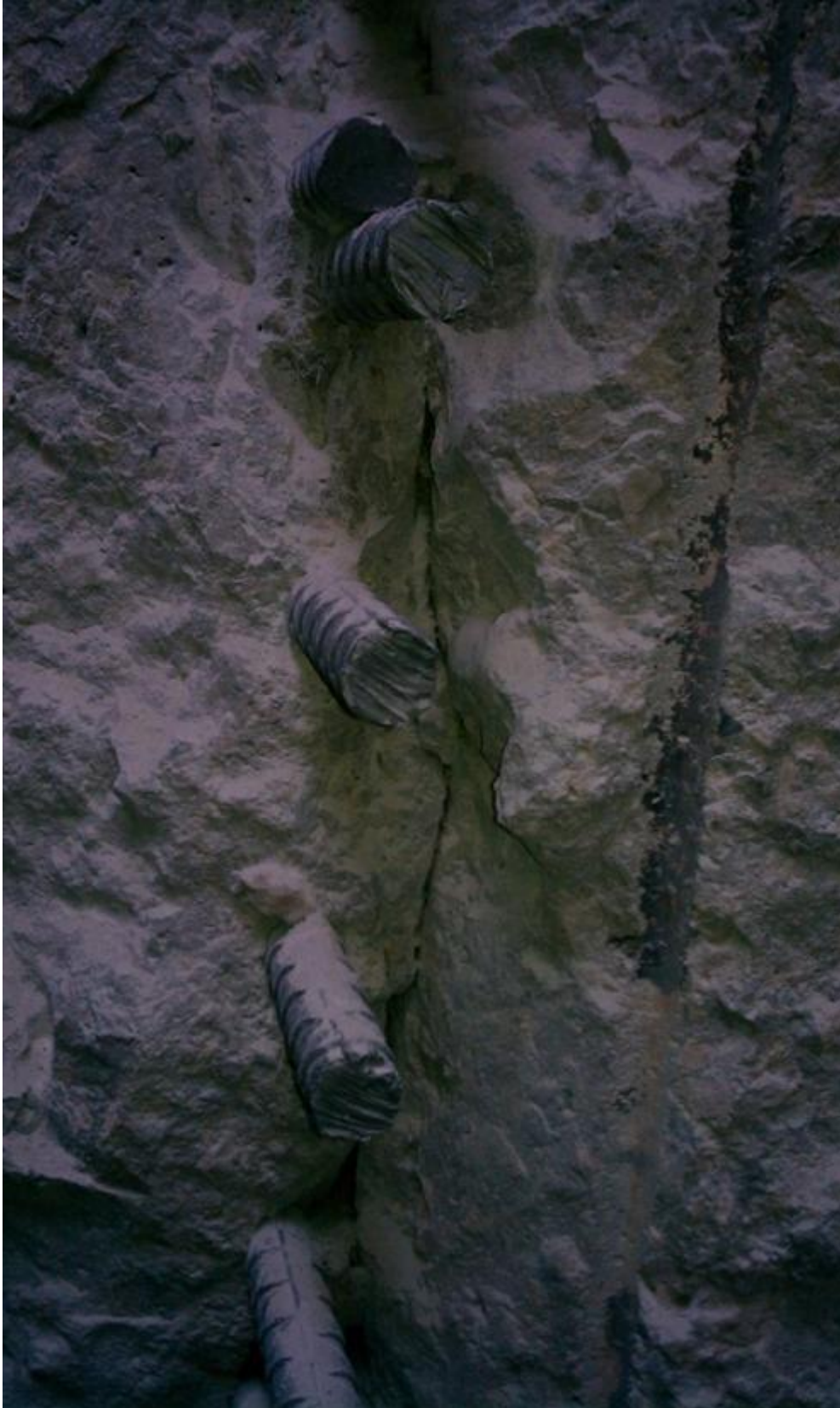
Picture No. 3 - Davis-Besse Shield Building Laminar Subsurface Cracking
