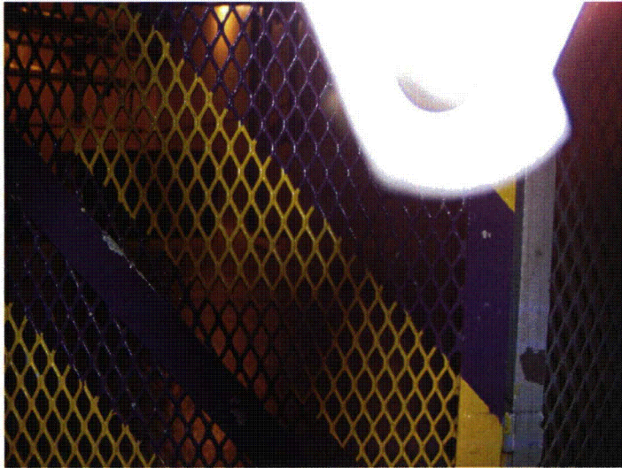
Figure 3e.1.1-2: Wire Mesh Door in Bioshield Doorway
