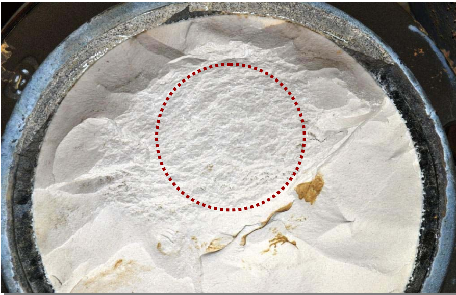
Unit 2 Failed Insulator
