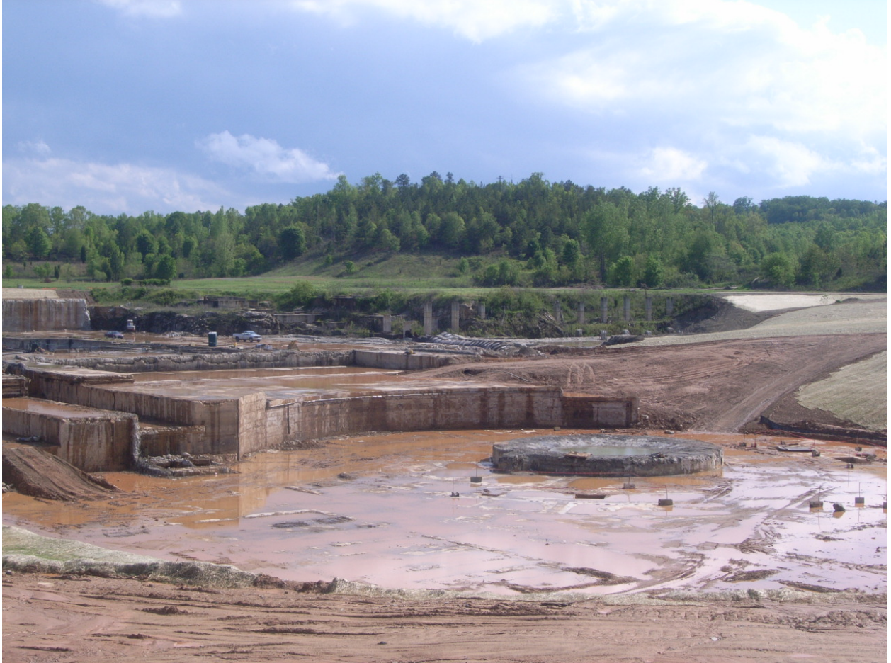
Figure 4. April-May 2008 Lee Nuclear Site Field Audit: View of concrete poured during initial construction activities at CNS Unit 1 (Lee Nuclear Site Unit 1).
