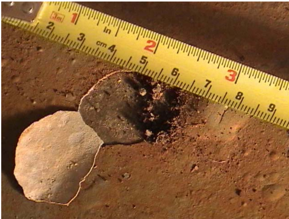
Figure 19. Floor coating failure on below-grade concrete, typical of moisture vapor transmission
