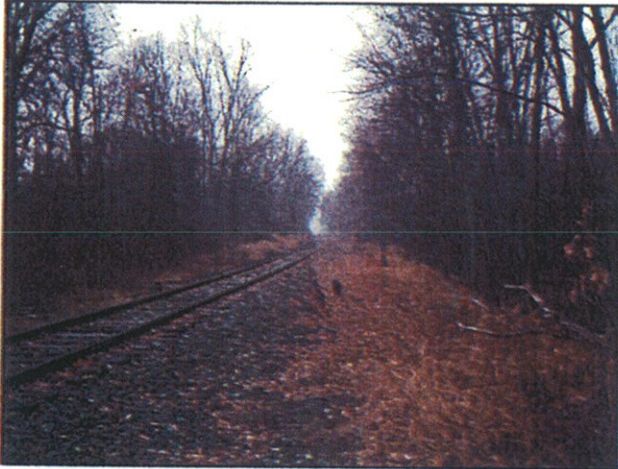
GAI-11 (155053) – The Bloomsburg Division of the Delaware, Lackawanna & Western Railway (Determined Not Eligible by PHMC)
