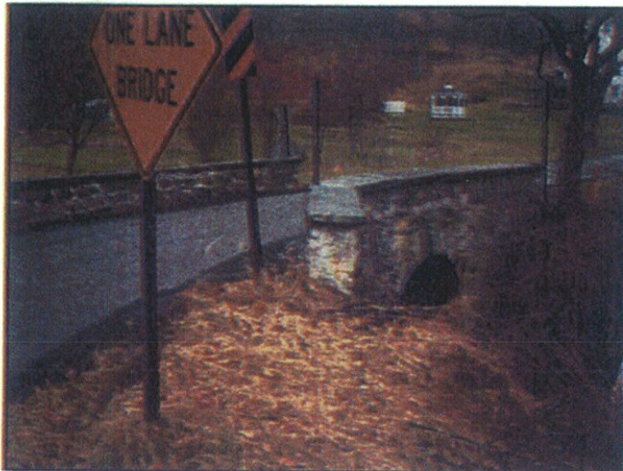
GAI-06 (155054) – Stone Arch Bridge, Beach Grove Road at Stone Church Road (Recommended Potentially Eligible)
