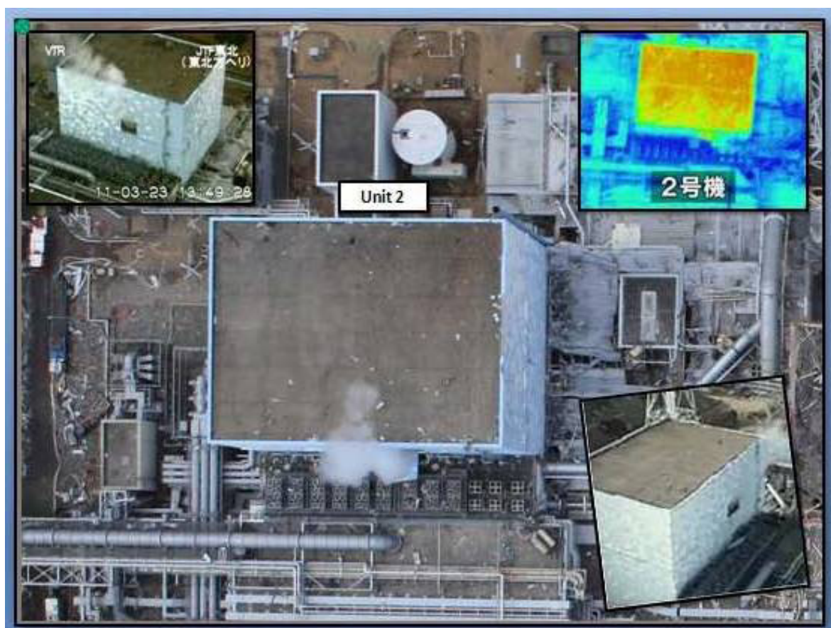
Figure 4: Damage to Unit 2
