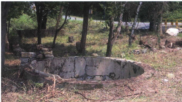
Photograph 14-7. Site 36LU283: Feature 2, Base of Concrete Silo, View to Southeast. Note Piers and East Foundation Wall in Background, Facing East
