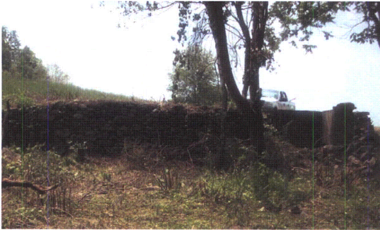
Photograph 14-8. Site 36LU283: Feature 2, West Foundation Wall Illustrating Concrete Foundation Attachment for Silo on Right, Facing West
