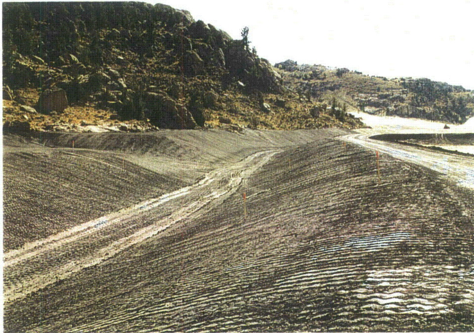
Photo 30 – South Diversion Ditch - Approx. Sta. 5+00 looking southeast at compacted radon barrier and confluence no.1, September, 1996
