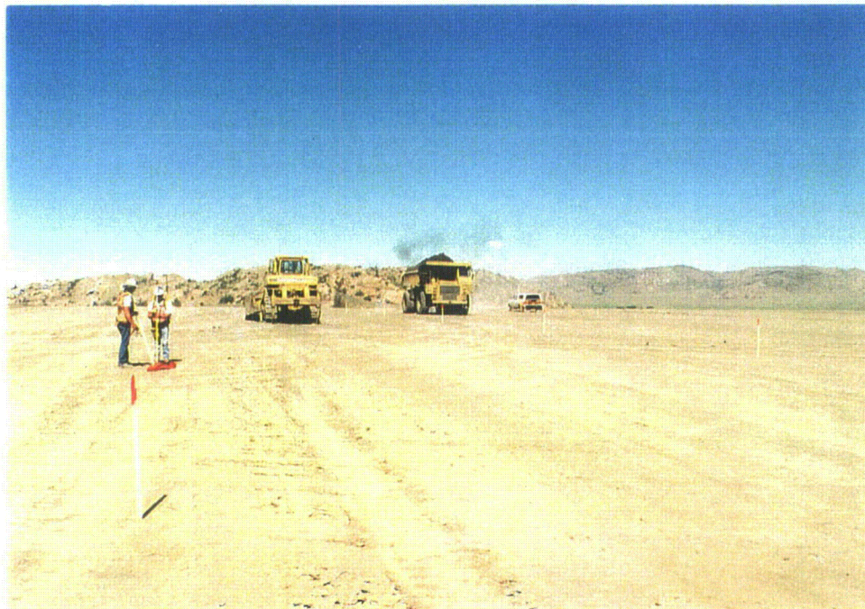
Photo 7 – Area 1B – Completed subgrade, GPS surveying for design elevation and beginning to haul Cody Shale clay for sacrificial clay layer, July, 1996
