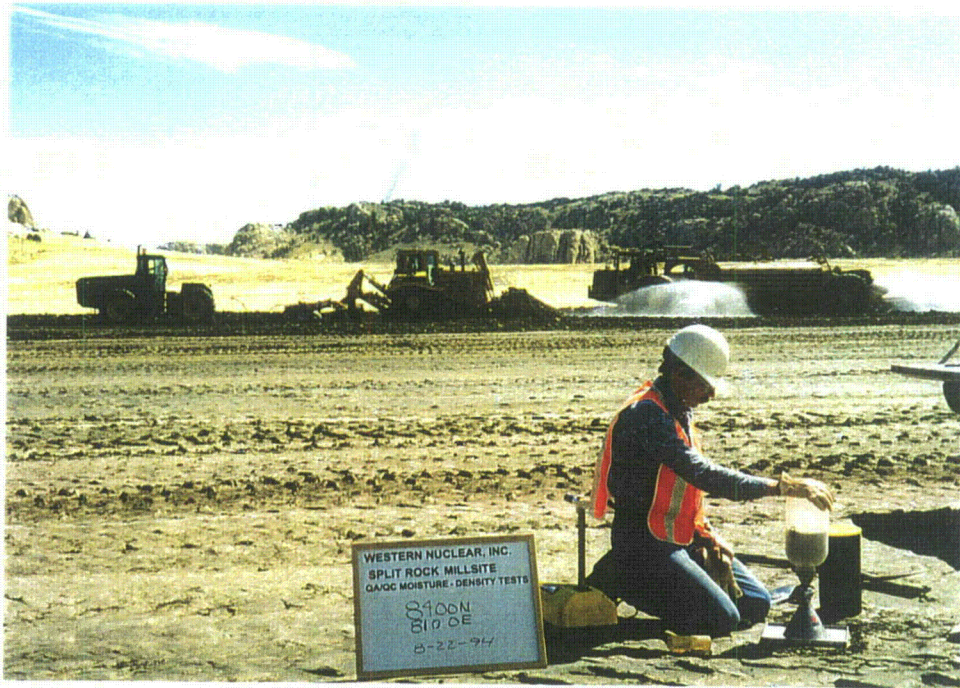
Photo 18 - Area 3A - Spreading clay - Disk processing clay - Spraying water, sand cone density testing in foreground, 1994
