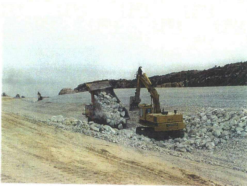
Photo 37 - Placing D_{50}18'' riprap in South Diversion Ditch at approximately station 32+00 and at approximately station 37+00, November, 1997
