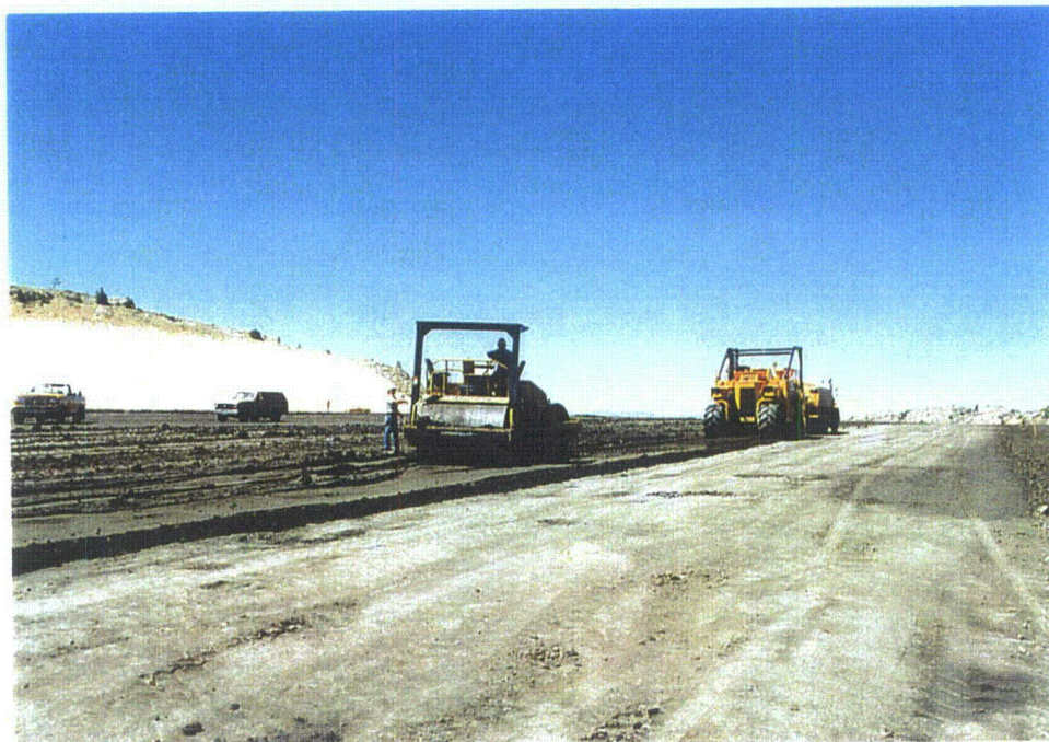
Photo 13 - Area 1A - Soil stabilizer processing clay for radon barrier and double drum vibratory roller compacting radon barrier, July, 1996
