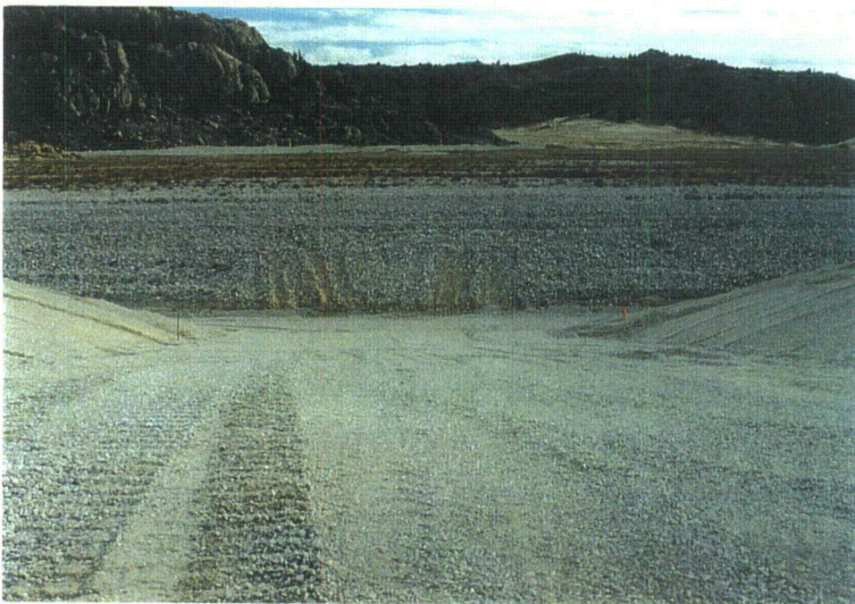
Photo 40 - Filter in confluence 4 North Diversion Ditch, September, 1998
