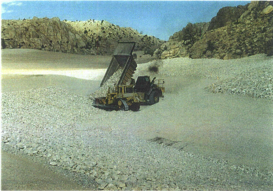
Photo 36 – South Diversion Ditch approximately station 15+00 looking east at placement of D_{50}3'' riprap over Filter I. D_{50}6'' rock mulch above and to right at juncture with rocks, October, 1996
