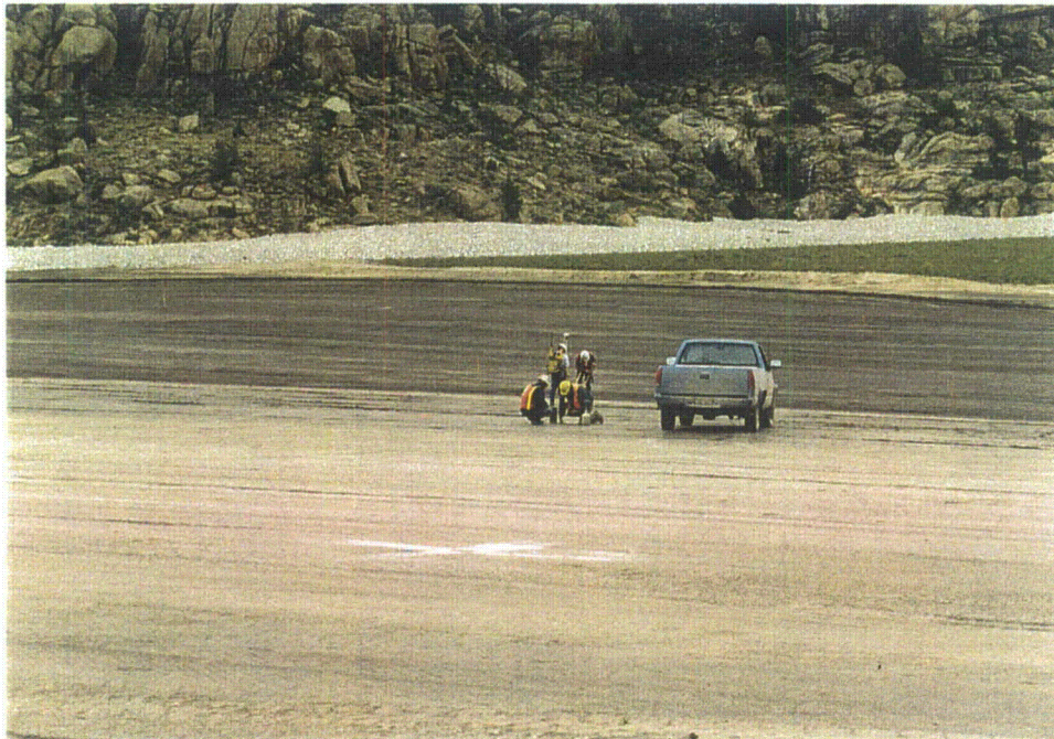
Photo 12 – Moisture Density testing radon barrier in swale and GPS survey locating test – Area 1A – North, September, 1997
