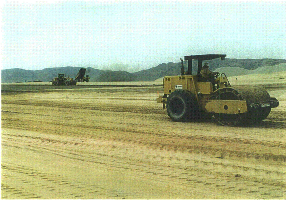
Photo 6 - Proof rolling subgrade surface and regraded areas of Area 1A prior to sacrificial placement, May, 1996
