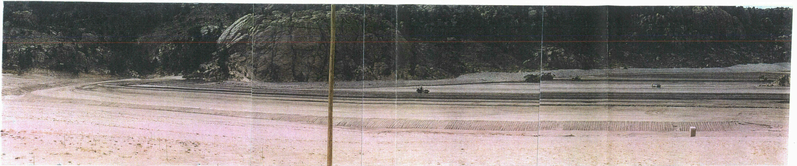
Photo 42 - Areas 2A, 2B, and 1C - Work almost complete - Looking Southeast to Southwest, November, 1995, (continued below)
