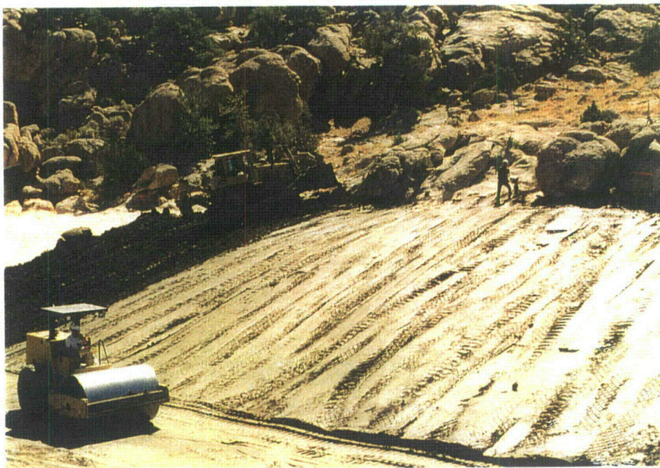
Photo 29 – South Diversion Ditch - Sacrificial clay and first lift - Approximately station 9+00 - Outside slope. Note hand compaction around granite outcrops, August, 1996
