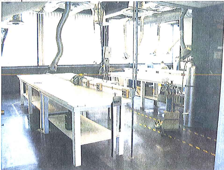
Figure 7. Room 1219 showing the flexible ducts referred to in this report. None of these ducts were contaminated.
