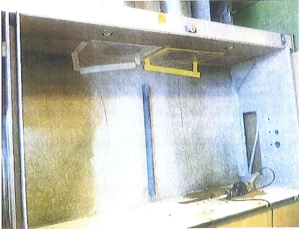
Figure 5. Interior of an 8-foot fume hood (Room 1205) with most of the metal components removed. The Transite® (asbestos) side panel as well as all the gas fittings has been removed. The clean area in the back shows that decontamination has been attempted. Non-abrasive decontamination of the Transite material was largely unsuccessful.
