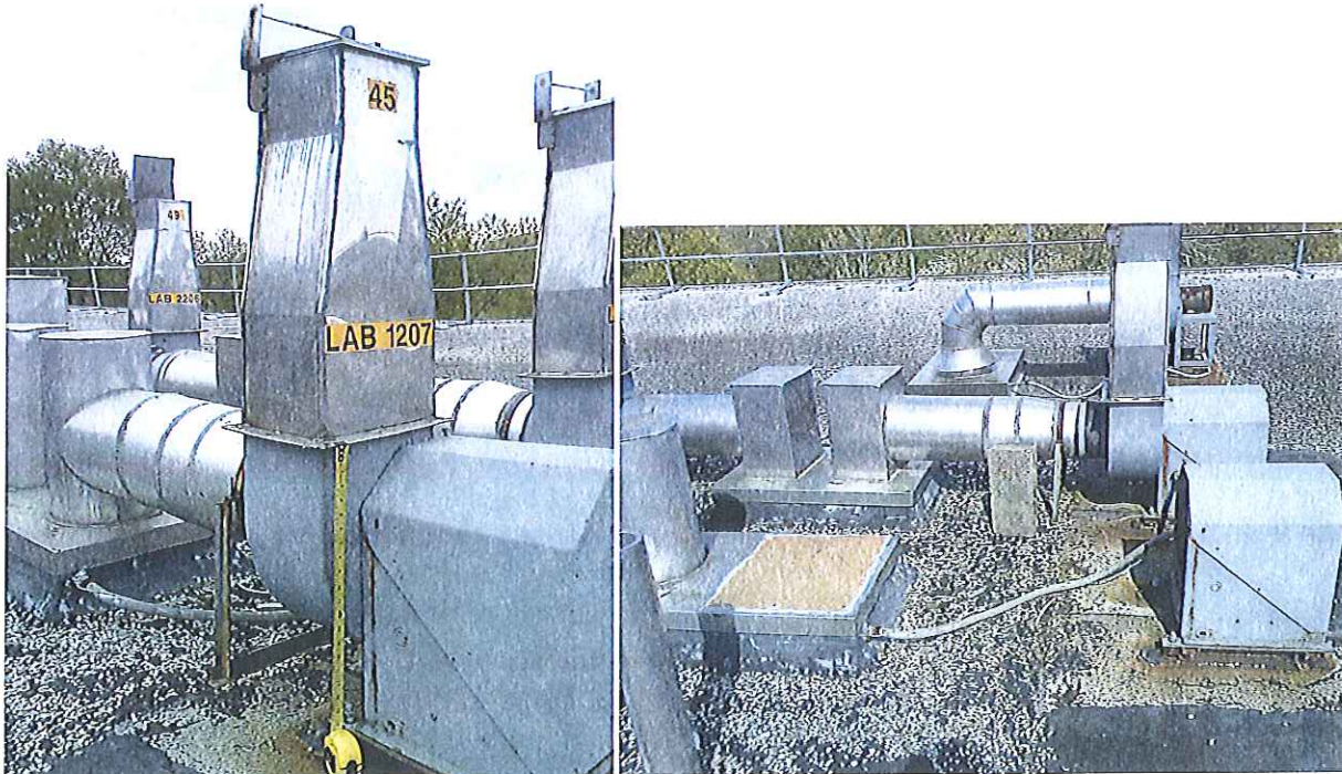
Figure 6. Roof-top ventilation ducting, blower and chimney for hood #45 in Room 1207 (left). Photo on right shows that the blower and ducting have been removed. The motor was not contaminated and was not removed.
