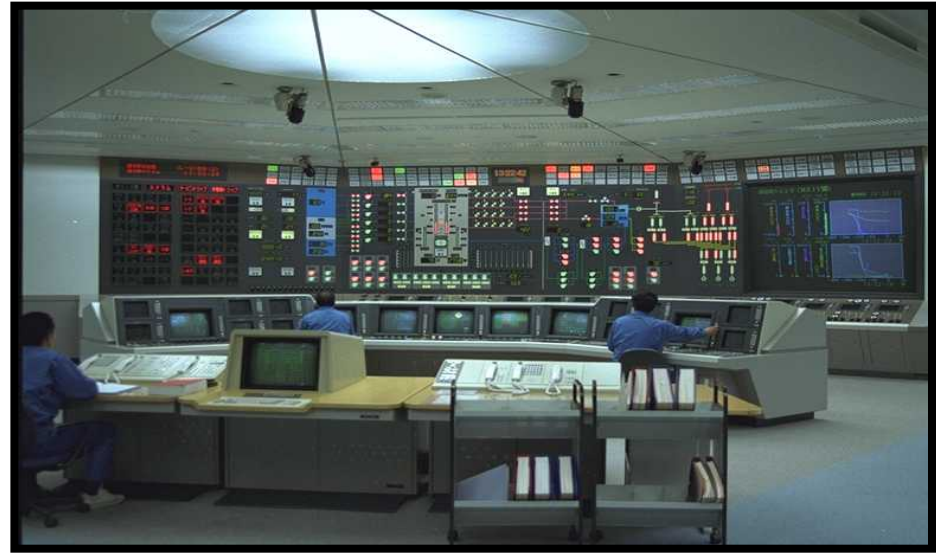
Control Room with Computer-based HSIs
