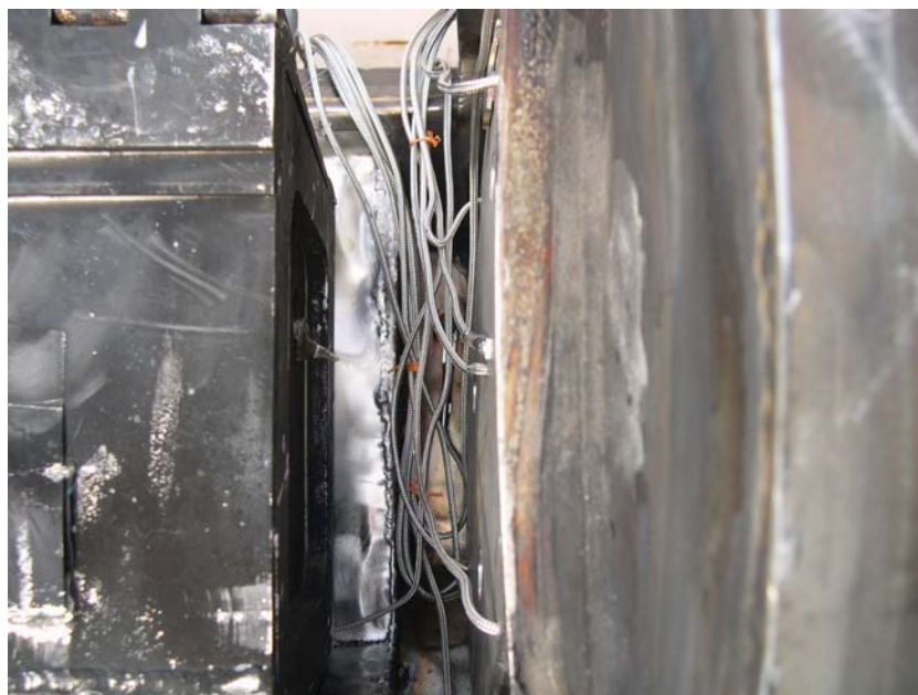
Figure 3-23 Outerpack Internals after December 15 Burn Test
