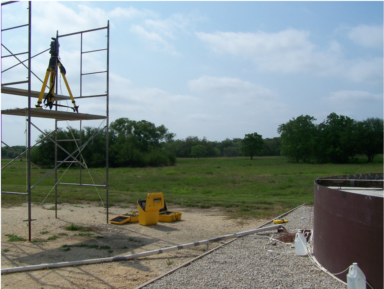
Figure 4-1. A Scaffold-Mounted Laser Scanner at the East End of the Intermediate-Scale Grout Monolith Was Used To Measure Surface Topography
