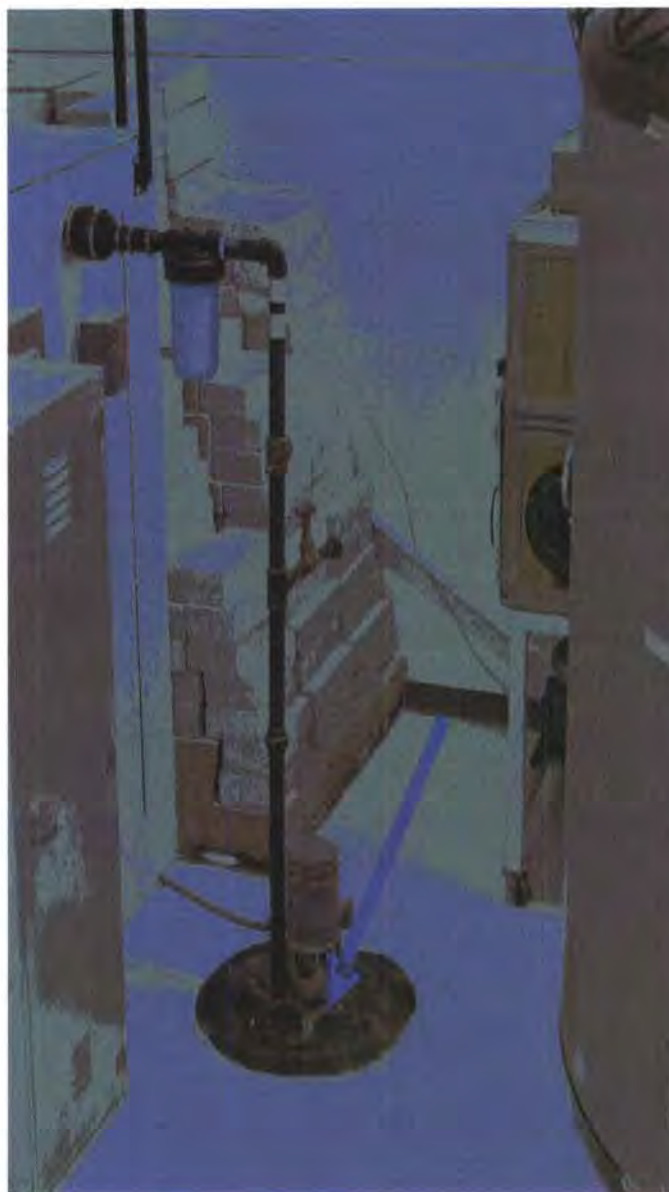
Figure 5.4-5 A 40-gallon water storage (indicated by arrow)
