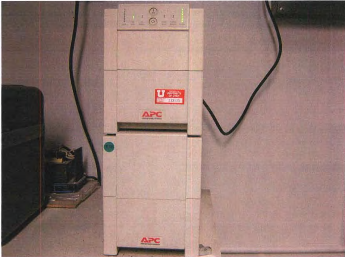
Figure 8.2-1 Uninterruptible Power Supply (UPS) for emergency electrical power
