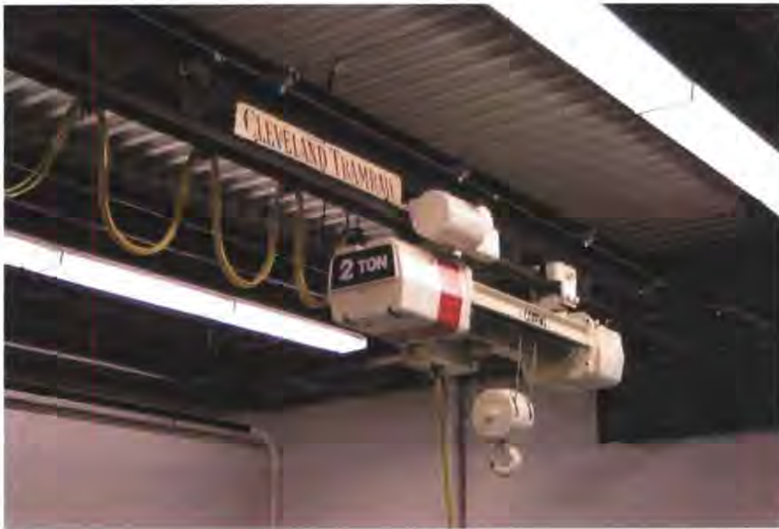
Figure 9.2-1 The UUTR overhead crane system
