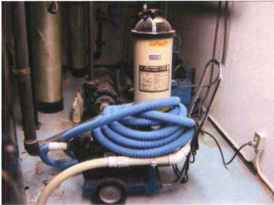
Figure 5.4-1 Under water cleanup system
