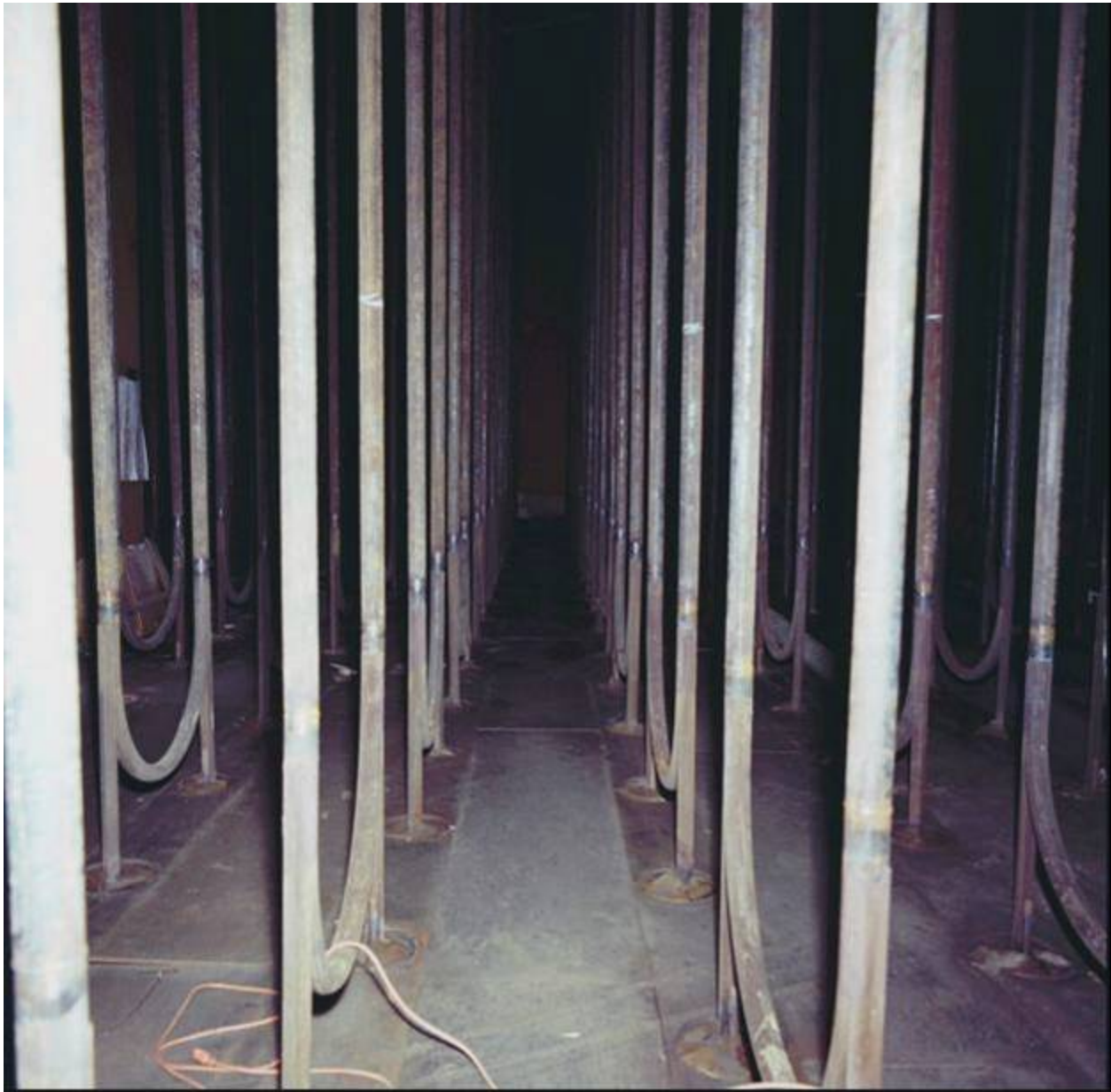
Figure 3.2-29: Cooling Coils in a Type IIIA Tank
