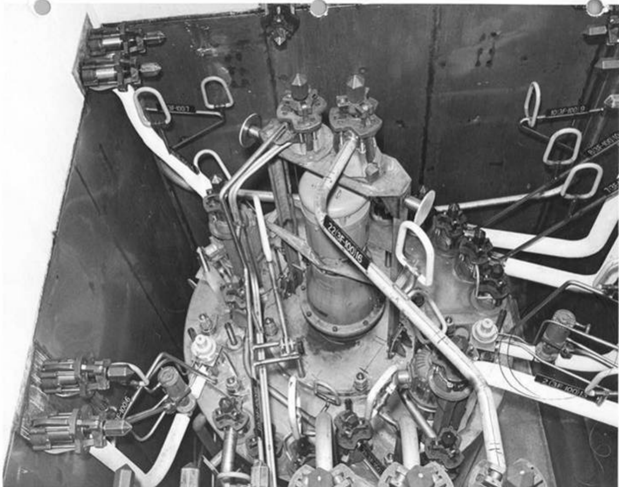
Figure 3.2-51: 242-F Evaporator CTS Pit and Tank
