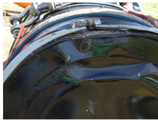
Close-up of Closure End Damage
