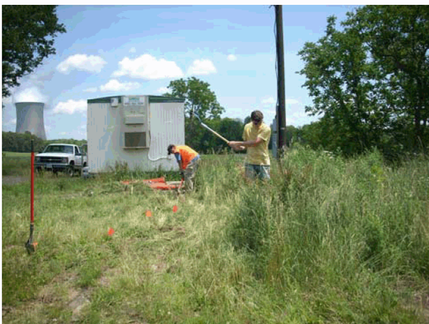
Photograph 24. Site 10 Showing Brush Clearing in Area of Former Structure 1, Work Trailer in Background, Facing East
