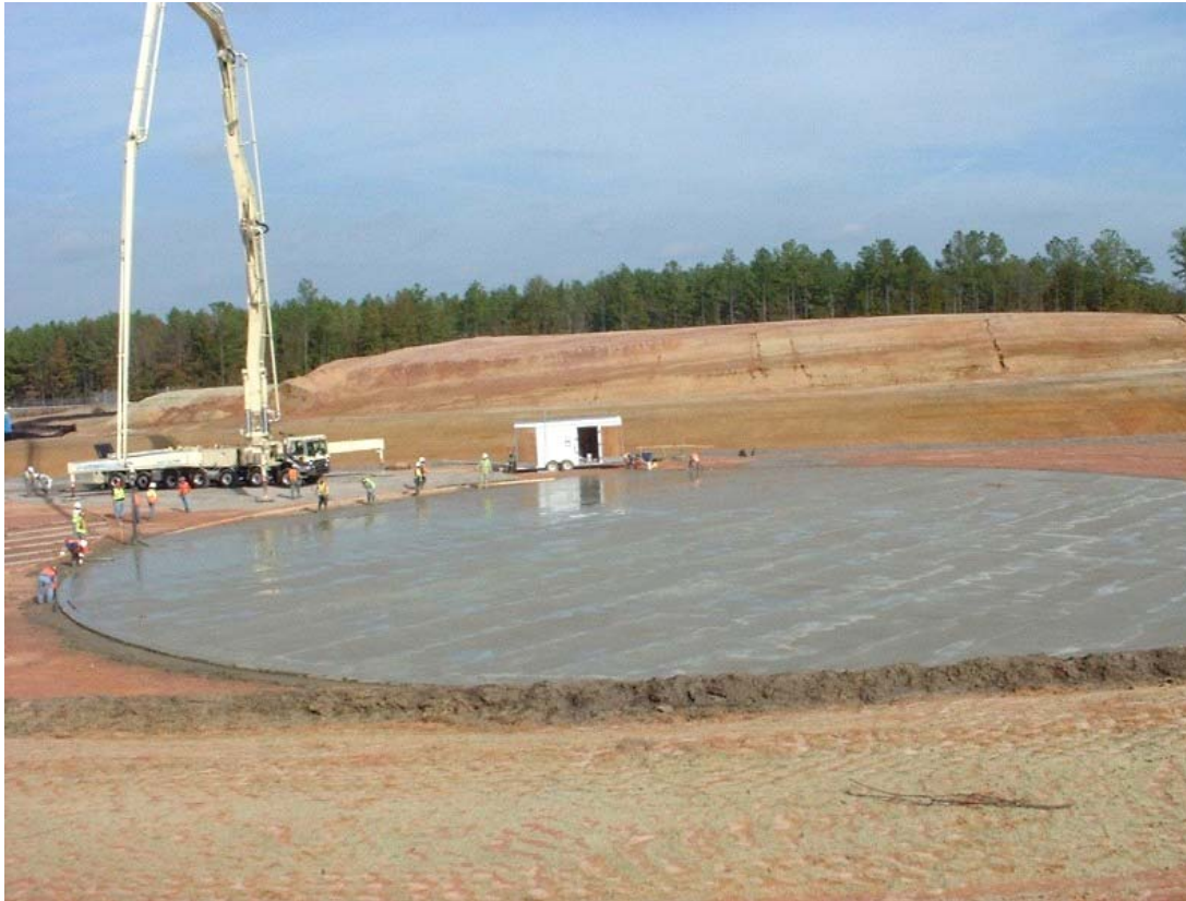
Figure 3.2-19: Placement of Lower Mud Mat for Disposal Unit 2 During Construction (Typical for FDCs)
