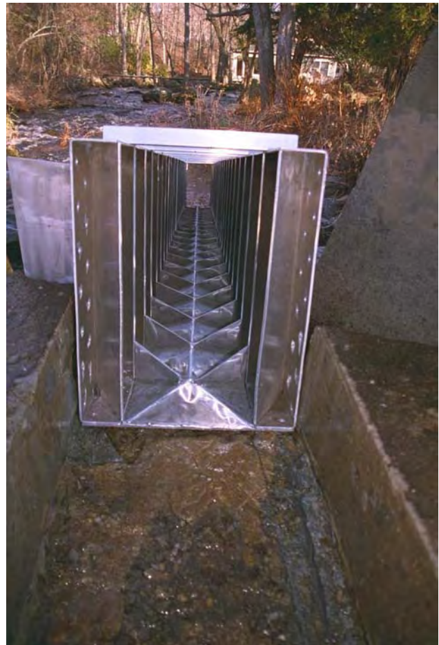
Fish bypass ladder installed on Parker River Dam, Byfield, MA, 2000. NOAA Restoration Center Community-based Restoration Project. Photo Credit: NOAA photo library.
