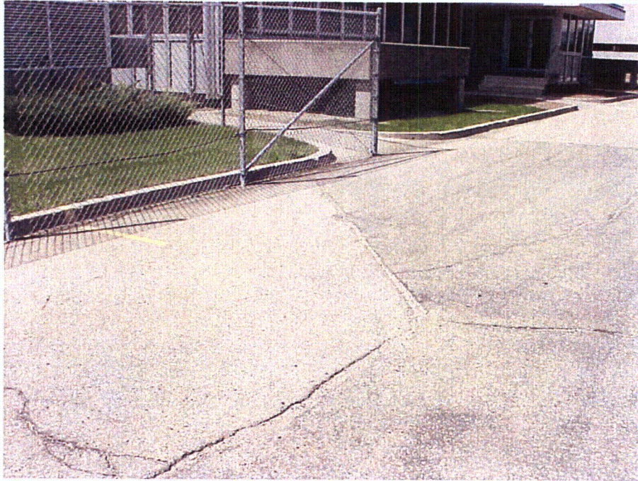
Photo 13: Photo of the truck unloading area for the 35,000 gallon Diesel Generator Fuel Oil USTs. Spill drainage from the area could reach Lake Michigan. Yellow line represents grade crest at truck unloading spot.
