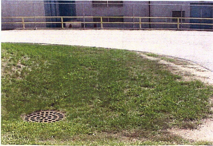
Photo 01: Storm grate in the truck unloading areas for the 10,000 gallon TSC Diesel Generator Fuel Oil UST.
