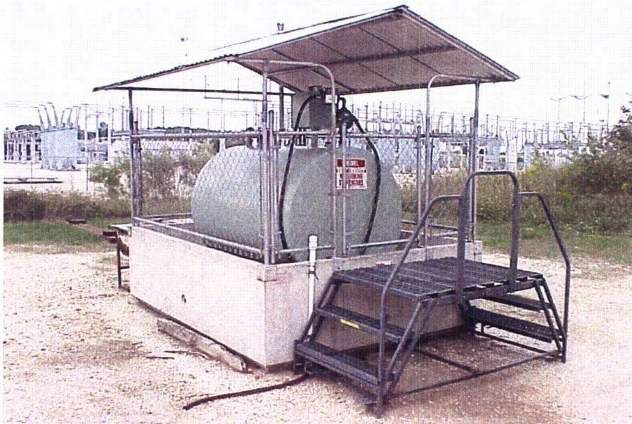
Photo 30: 600 Gallon Diesel Fuel STF/OTF Tank in Containment Dike with drainage hose in foreground.
