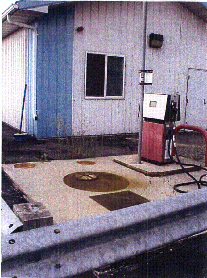
Photo 25: 550 Gallon Gasoline Dispensing UST Next to Vehicle Storage Building.
