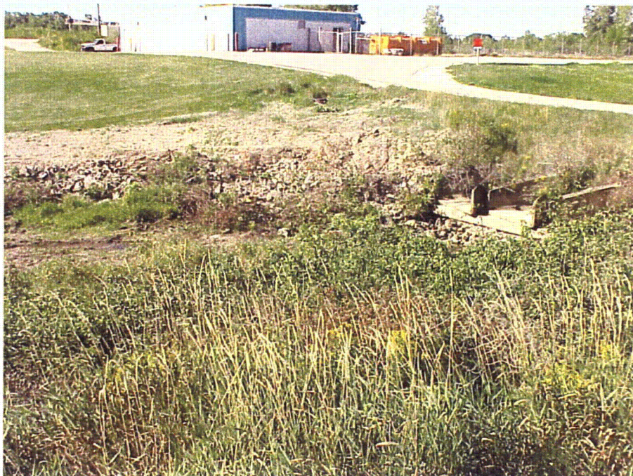
Photo 46: Tributary Ditch Serving Transformer Switchyard Runoff and Sewage Treatment Plant Treated Effluent
