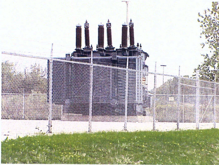
Photo 37: Uncontained Spare Dominion Main Transformer at Switchyard (Gravel Area Containment Only)
