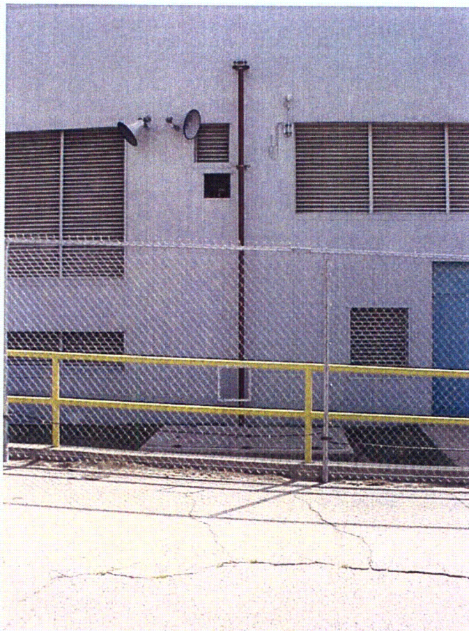
Photo 16: Photo of the truck unloading area for the 10,000 gallon TSC Diesel Fuel Oil Tank. Drainage would reach Lake Michigan stormwater drains.
