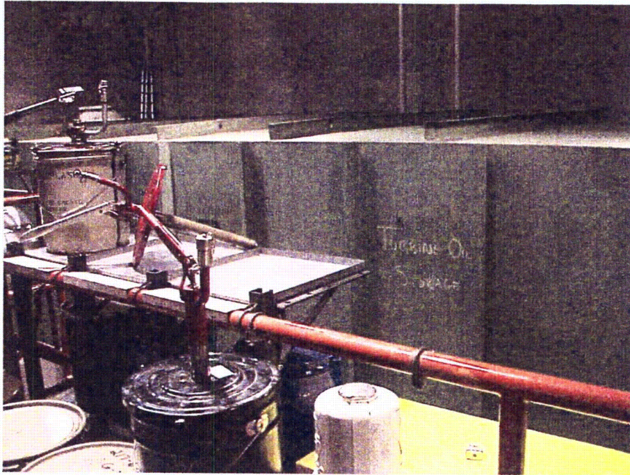
Photo 05: 14,000 Turbine Oil Tank Tank.
