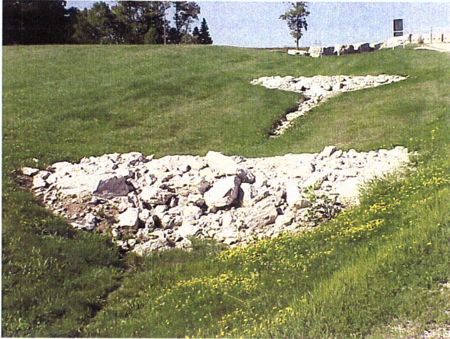
Photo 51: BMP Flow Restriction Measure from Runoff near Transformer Switchyard.
