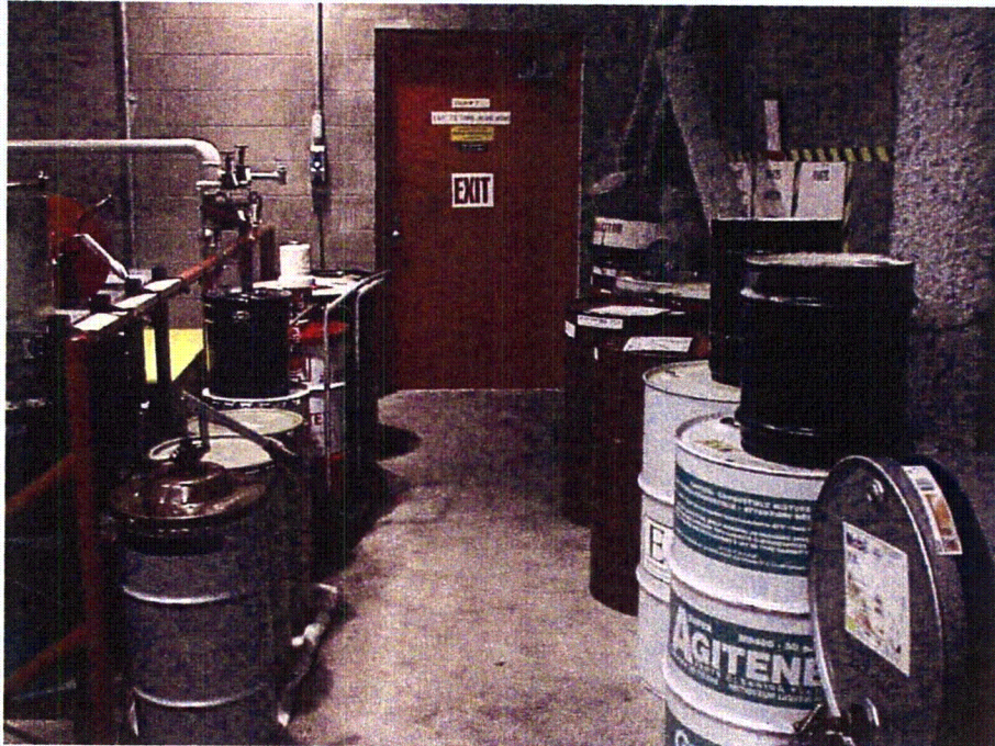
Photo 06: 14,000 Turbine Oil Tank room also has Drum Storage within room with curb at door.
