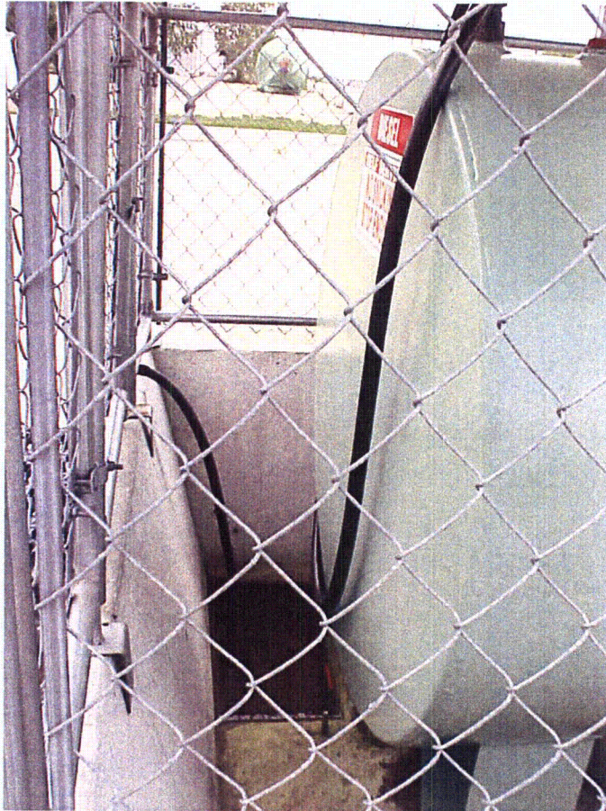
Photo 29: 600 Gallon Diesel Fuel OTF/STF Tank at Pump House
