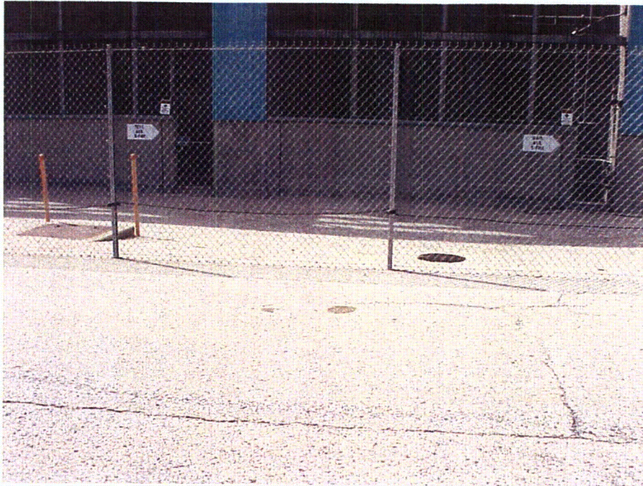
Photo 11: Photo shows Station Transformer area where a Lake Michigan stormwater drain is outside of containment. Trucks are utilized to transfer oil to or from a transformer in this area. The left side of photo shows drainage sump #2.
