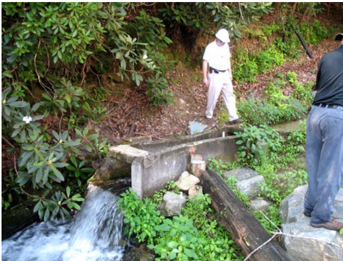
Clear discharge from a flume at the main seepage collection point low on the western abutment of Jocassee Dam.
