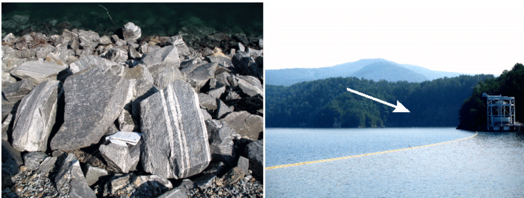
Upper left: Biotite gneiss (metamorphic rock) that serves as rip rap at Jocassee Dam. This rock type is extremely durable and not subject to breakdown over time under saturated conditions. Upper right: Arrow points to lake embayment that Duke representatives identified as the main quarry site (now submerged) used to obtain Jocassee Dam rock fill materials. Structure at right is one of two Jocassee intake structures.
