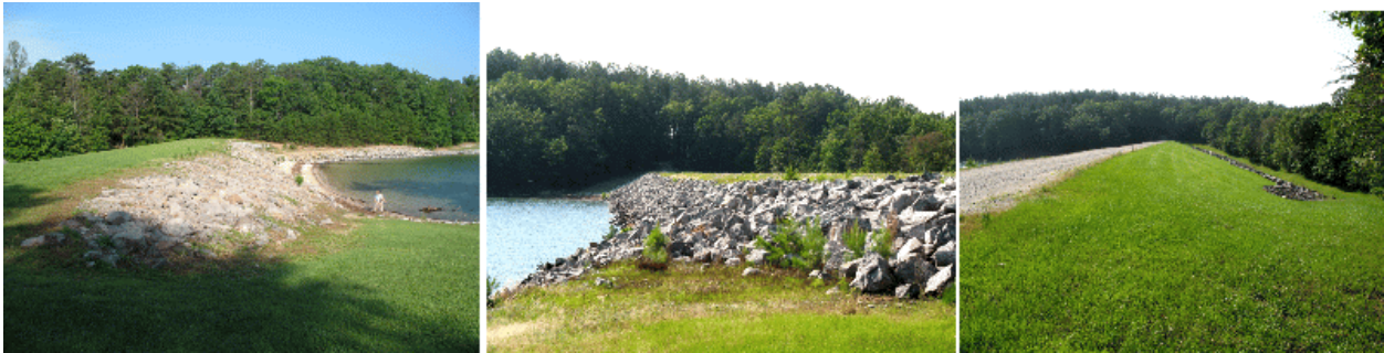
Saddle dikes at Jocassee Lake are protected from wave action by rip rap on sides facing lake. Top: Saddle Dike #2. Middle: rip rap on lake side of Dike #1. Right: downstream side of Dike #1 has grass but no rip rap (french drain is visible along toe of dam).
