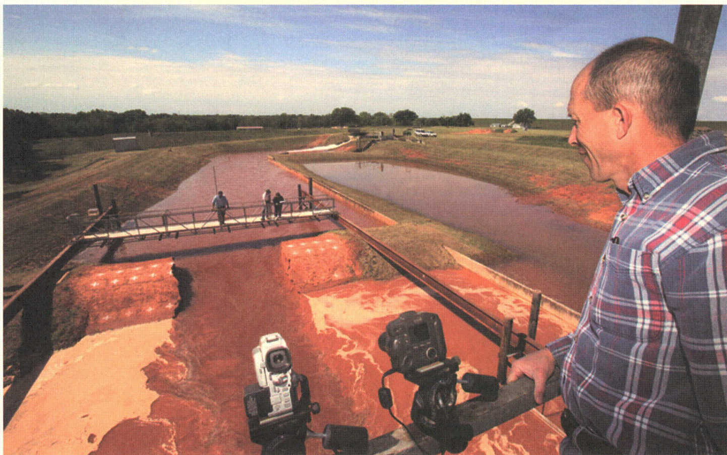
From an observation platform overlooking a test dam, hydraulic engineer Greg Hanson records the test for use in computer modeling. Photo courtesy of USDA, ARS, Stephen Ausmus.
