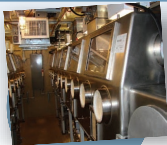
MOBILE GLOVEBOX FOR PLUTONIUM HANDLING
