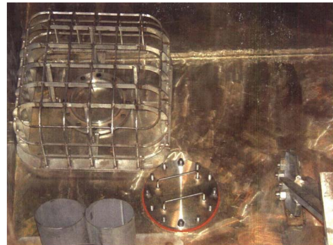
Figure 3I-1. Refueling Pool Trash Rack Cage
