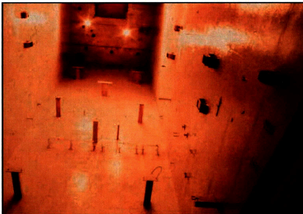
Figure 3-19. Extraction Cell 3 (After removal of processing equipment and before installation of the WVDP Liquid Waste Treatment System Equipment)
