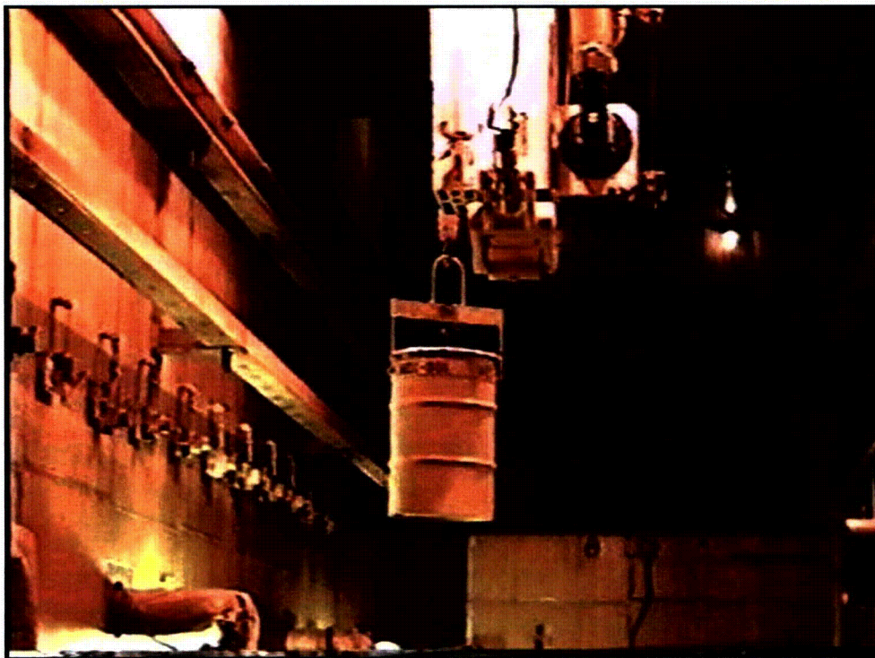
Figure 3-18. Process Mechanical Cell During Activation
