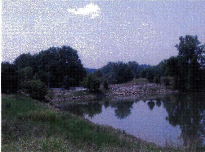
Figure 4: View of upstream side of dam with the concrete spillway. Note numerous trees that will need to be removed.
