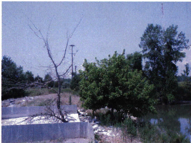
Figure 5: View of crest of dam and upstream edge of concrete spillway. A weir for measuring flow is located on the upstream end of the spillway.
