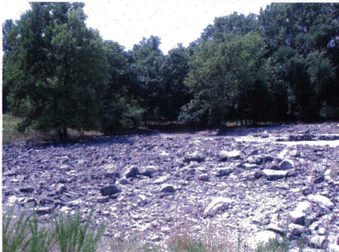
Figure 6: View of downstream slope of dam, with concrete spillway slab. Note trees located along the toe which will require removal.
