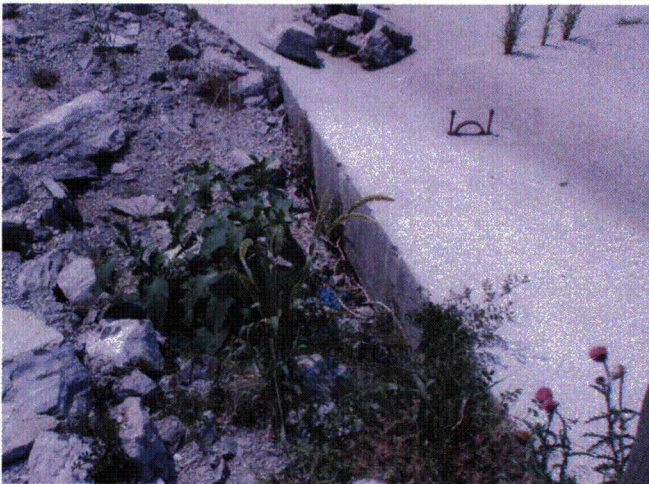
Figure 8: View of a small hole that has undermined the concrete spillway slab.
