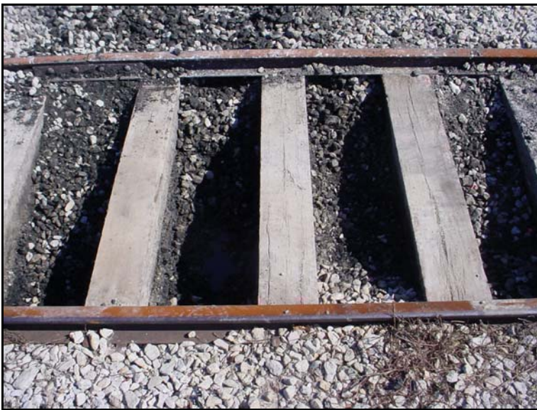
Scale Area. Material Removed from Between RR Ties
