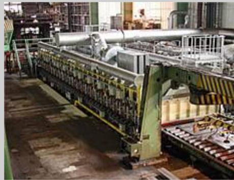
Continuous annealing furnace at the Siegen plant
