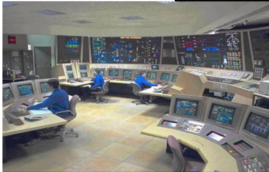
N4 Control Room
