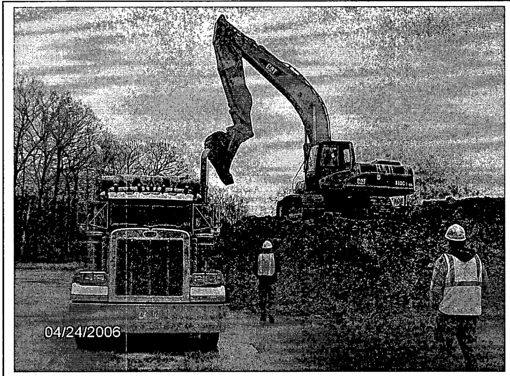
Day one of shipping waste staged on the pad begins. The schedule calls for fifteen truck loads a day carrying an average of 21.5 tons per truck.
