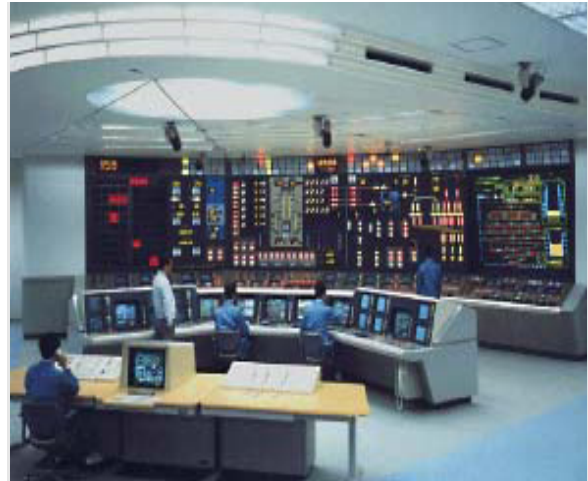
A Highly Integrated Control Room
