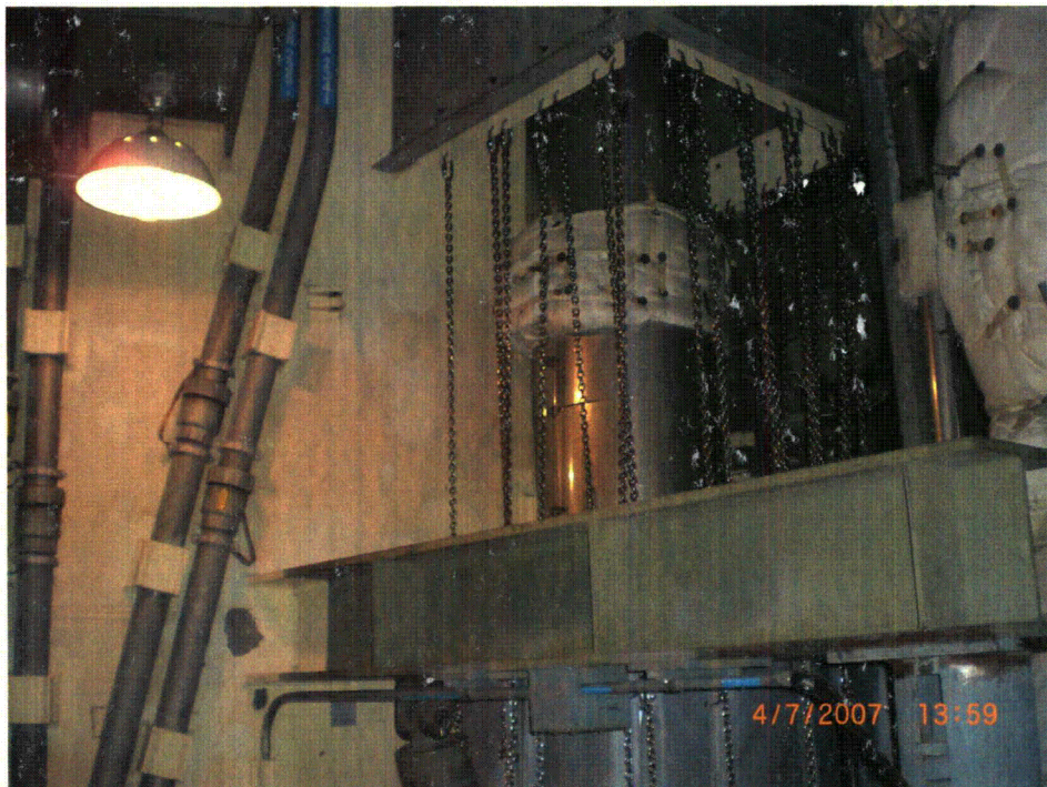
IR-055 Figure 6 Permanent Lead Shielding supported by the Jet Impingement Shield Assembly
