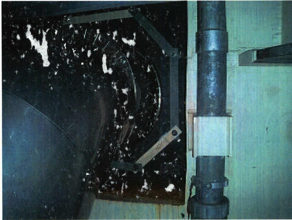
IR-055 Figure 4 View of N1A Bioshield Penetration with Shield Blocks in Place
