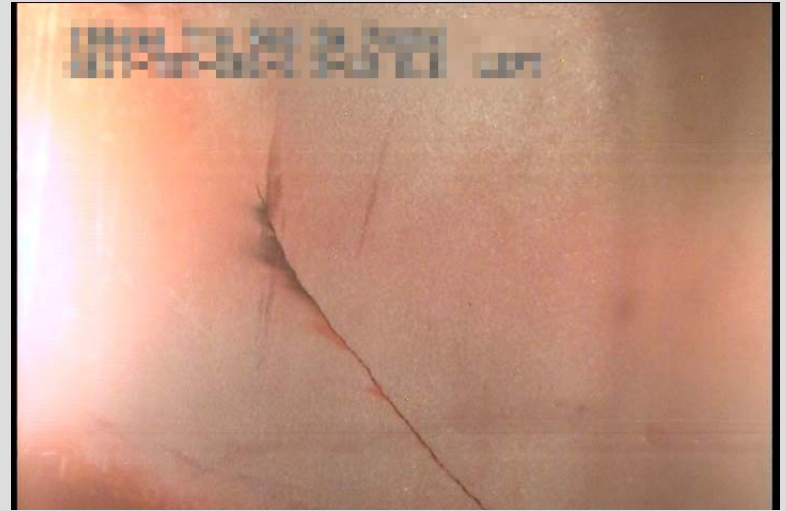
Discolorations at Crack Surface
