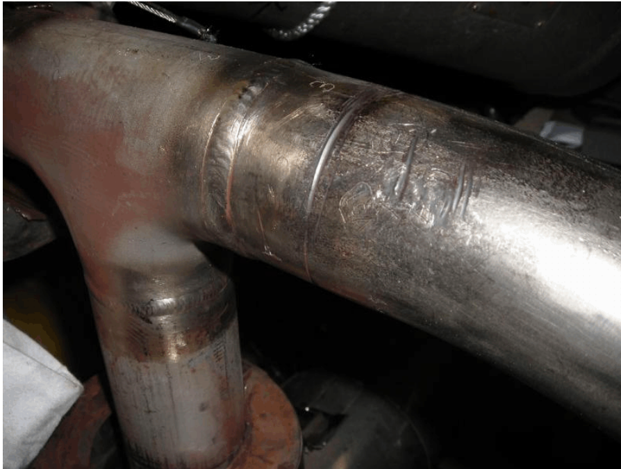
Figure 1: Wear indications identified on CVCS Letdown Piping
