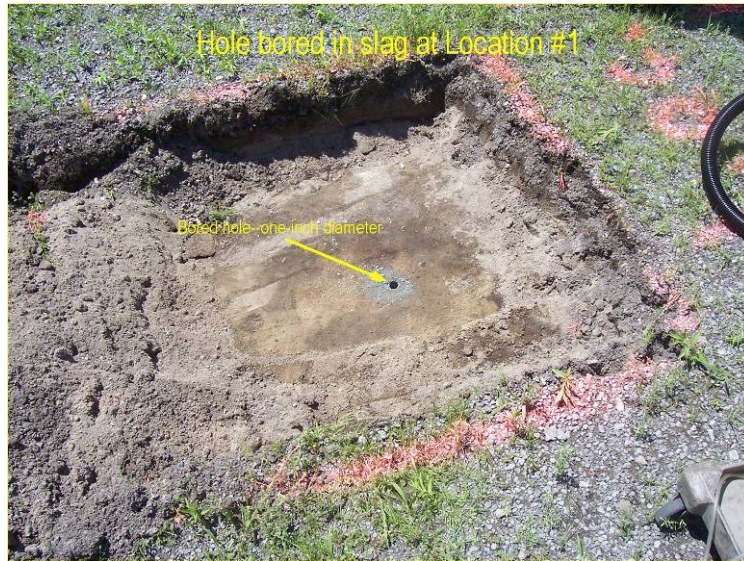
Figure 1: Hammond Monolithic Slag Layer, Overlying Soil Removed, AOC Southwest of Burn Cage
