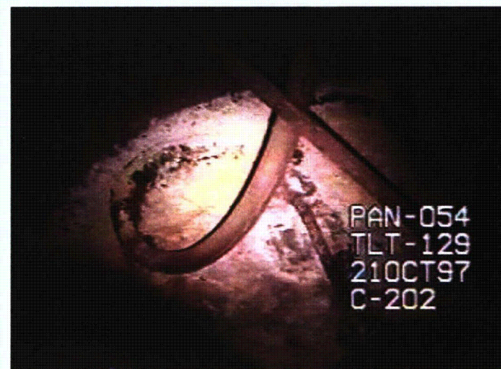
Abandoned Flex-Hose and Piping in Tank
