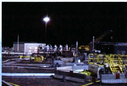
A well prepared and rehearsed team of skilled tank farm workers installed the Off Riser Sampling System (ORSS) in single-shell tank C-103. The device is capable of moving around inside a tank and improves our capability to obtain residual waste samples in locations not accessible beneath access risers.
