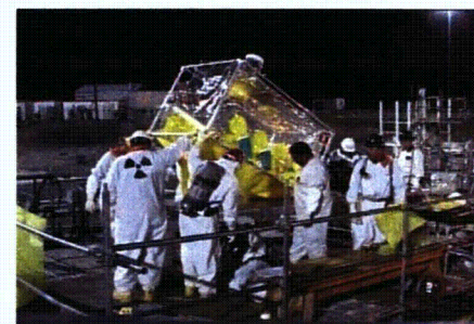
Once ready to be lowered into the tank a glove bag is installed to contain any potential contamination and still give workers access to the equipment.
