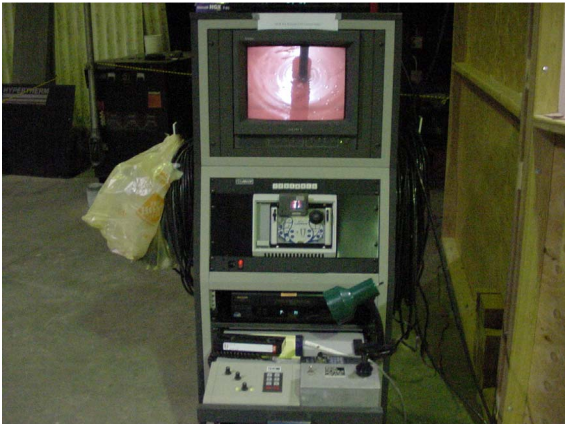
Figure 5. Video camera system remote operation and video recording system.
