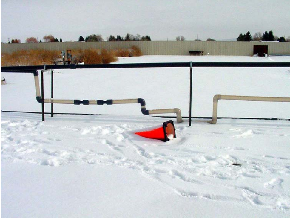
Figure 3. Slurry Pipe Configuration
