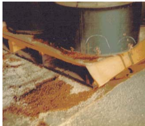
Figure 6 – Compromised Storage Drum
