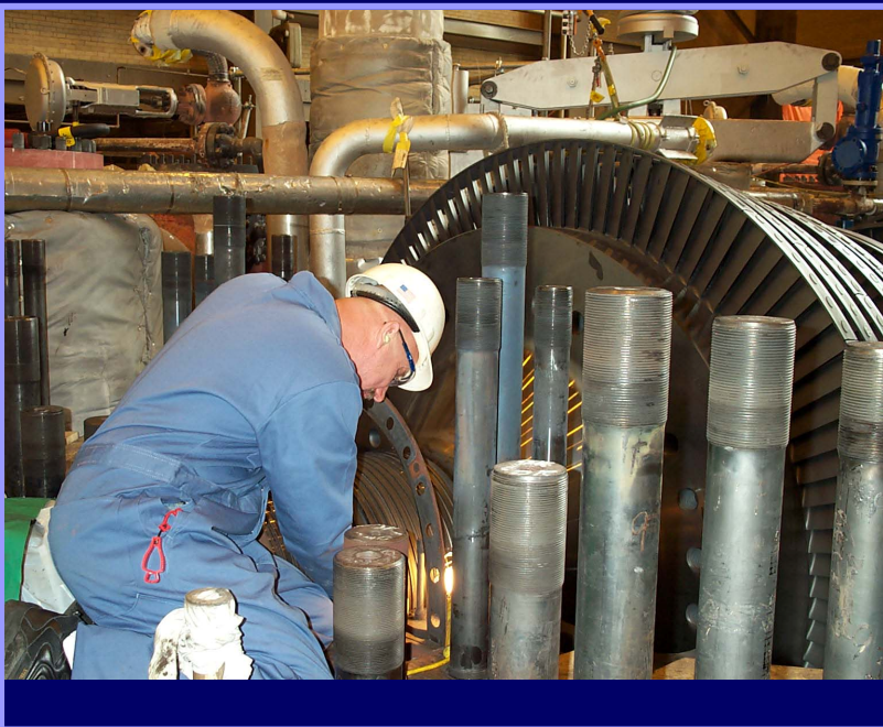
New HP Turbines
